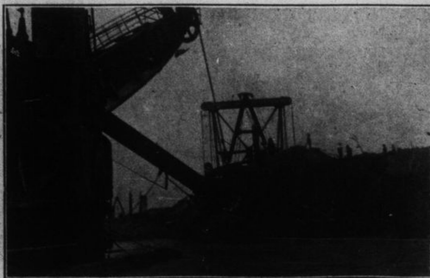
Latest photograph from the Canal, showing the huge dredge at work removing the earth that has closed the slide for so long a time.
