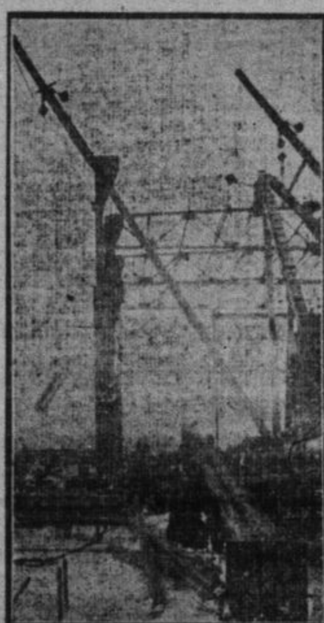
Travelling Derricks at Work, Finishing End Span of Boiler and Tank Shop.
