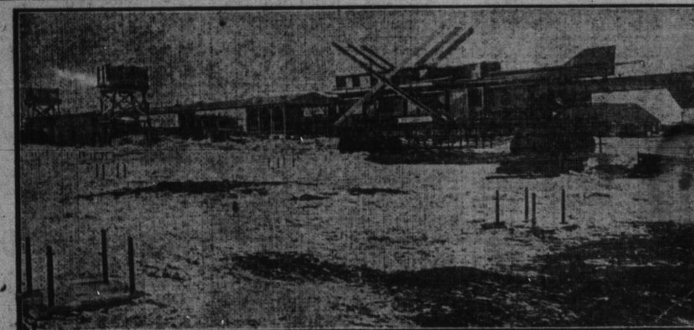
North of Locomotive Shops—Concrete Foundation for Columns for the Frog and Track Shop—Car of Steel Ready to Unload.
