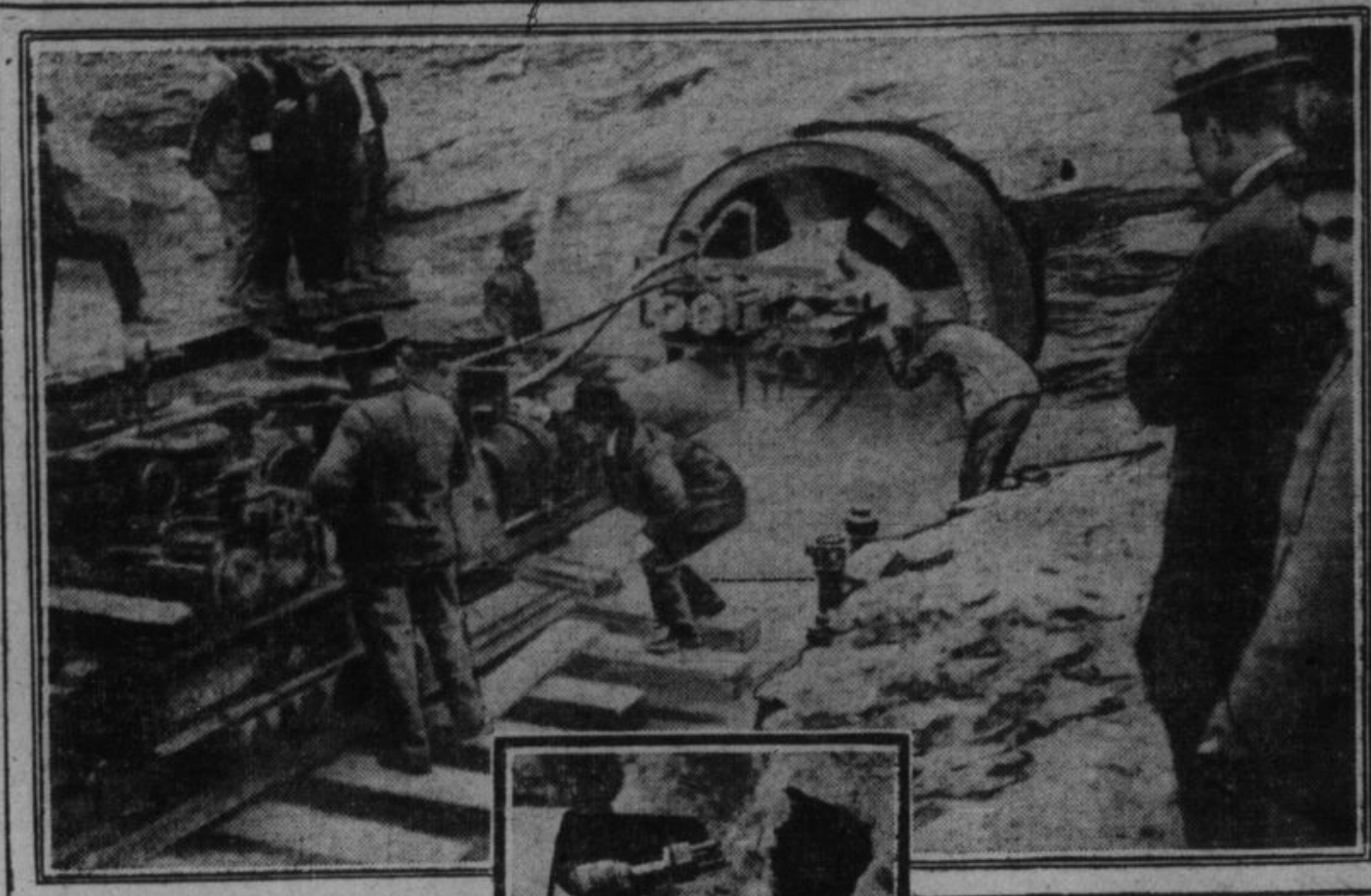
TERRY, TRENCH AND PROCTOR'S TUNNELLING MACHINE AT WORK IN GRAND CENTRAL YARDS.
