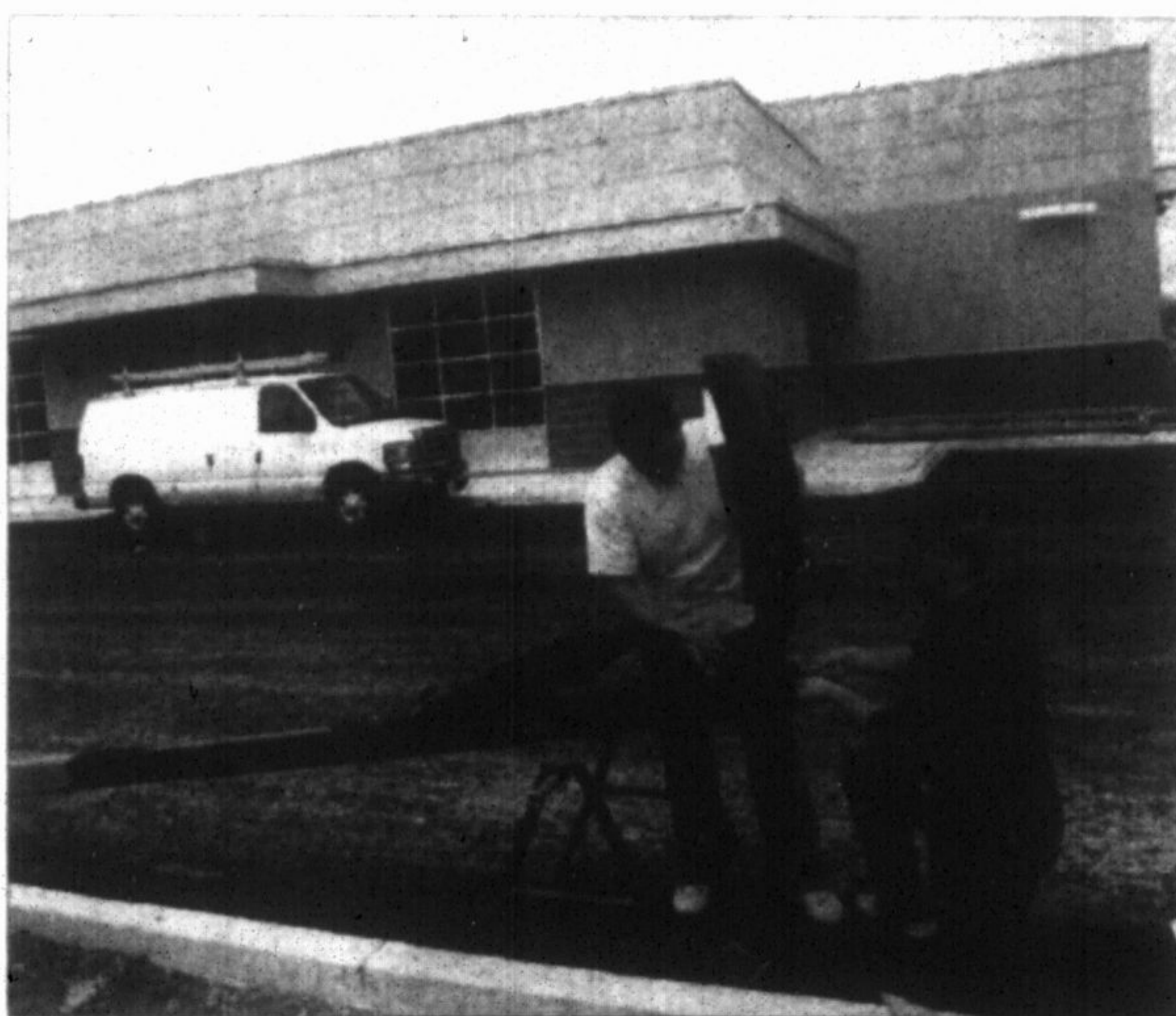
Rob Bolzicco (left) and Mike Massi of Dur Electric work on an outdoor light at the new Royal Canadian Legion Thursday.
