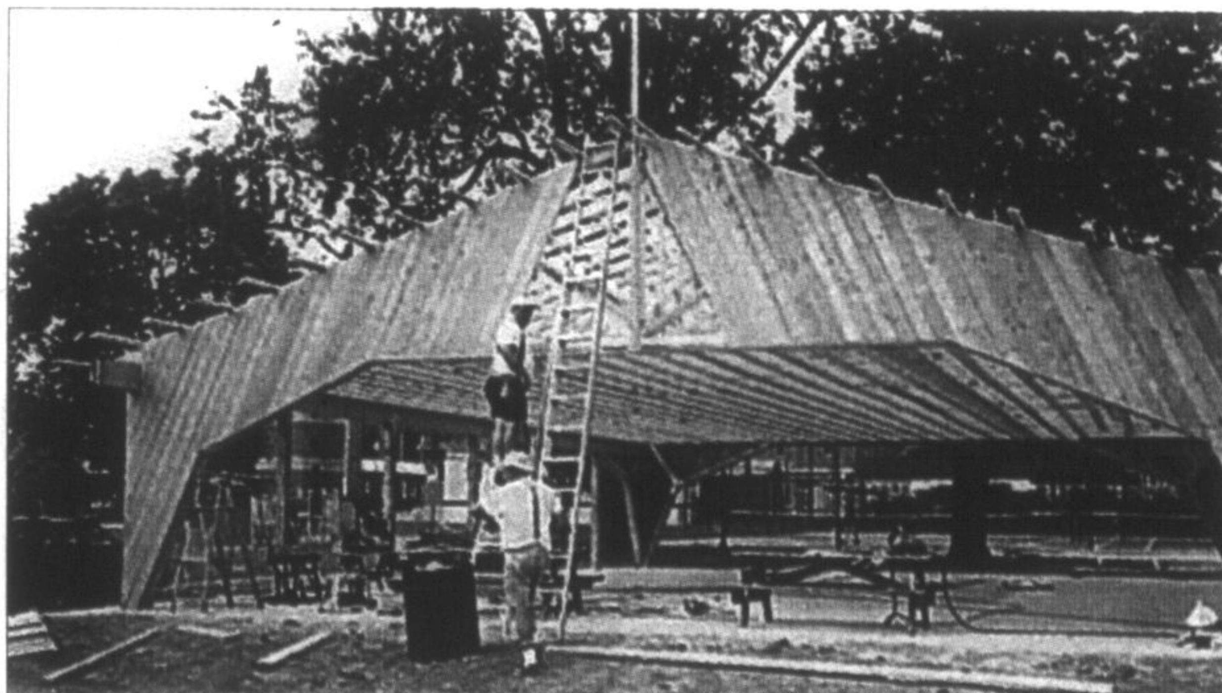
Club members work on the reconstruction of the Memorial Park pavilion in 1998.
