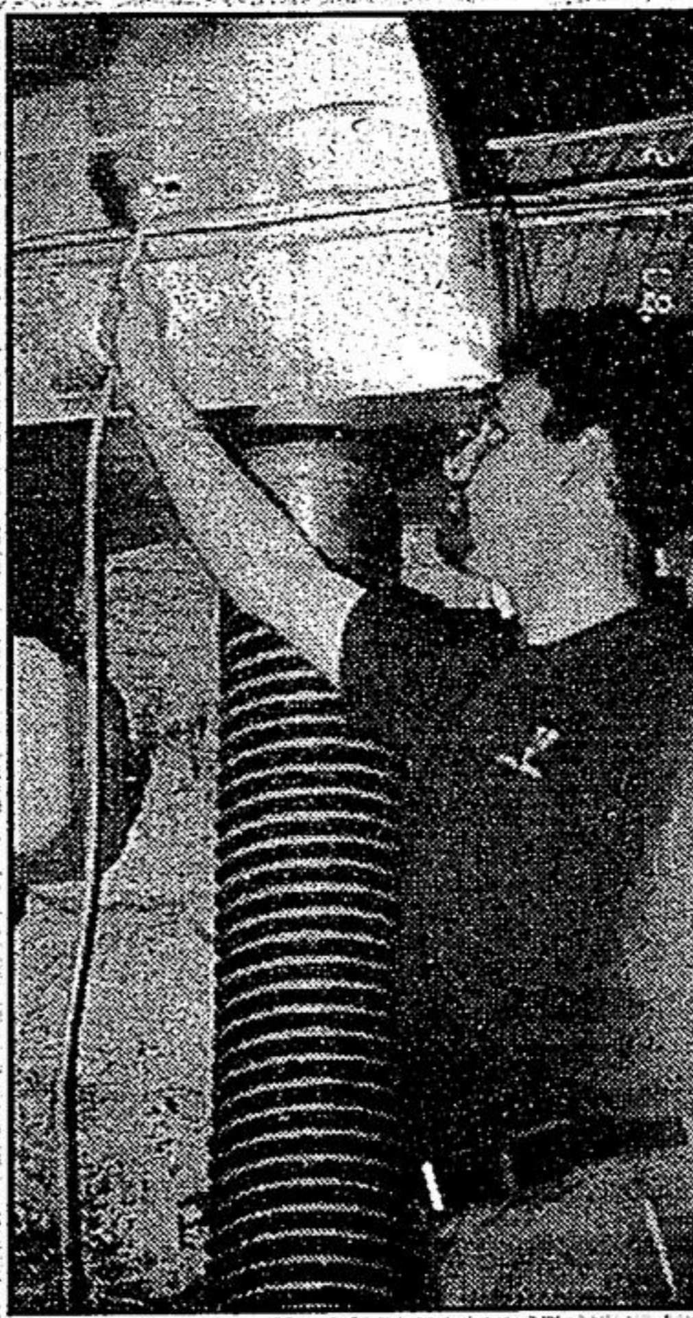
V Care provides a number of services including duct cleaning.
