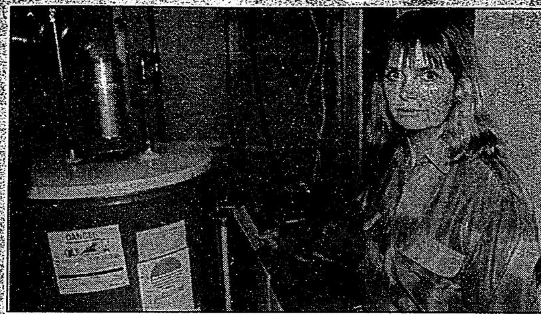
Judy Smith shows the tag which indicates regular service is mandatory on water heaters.
