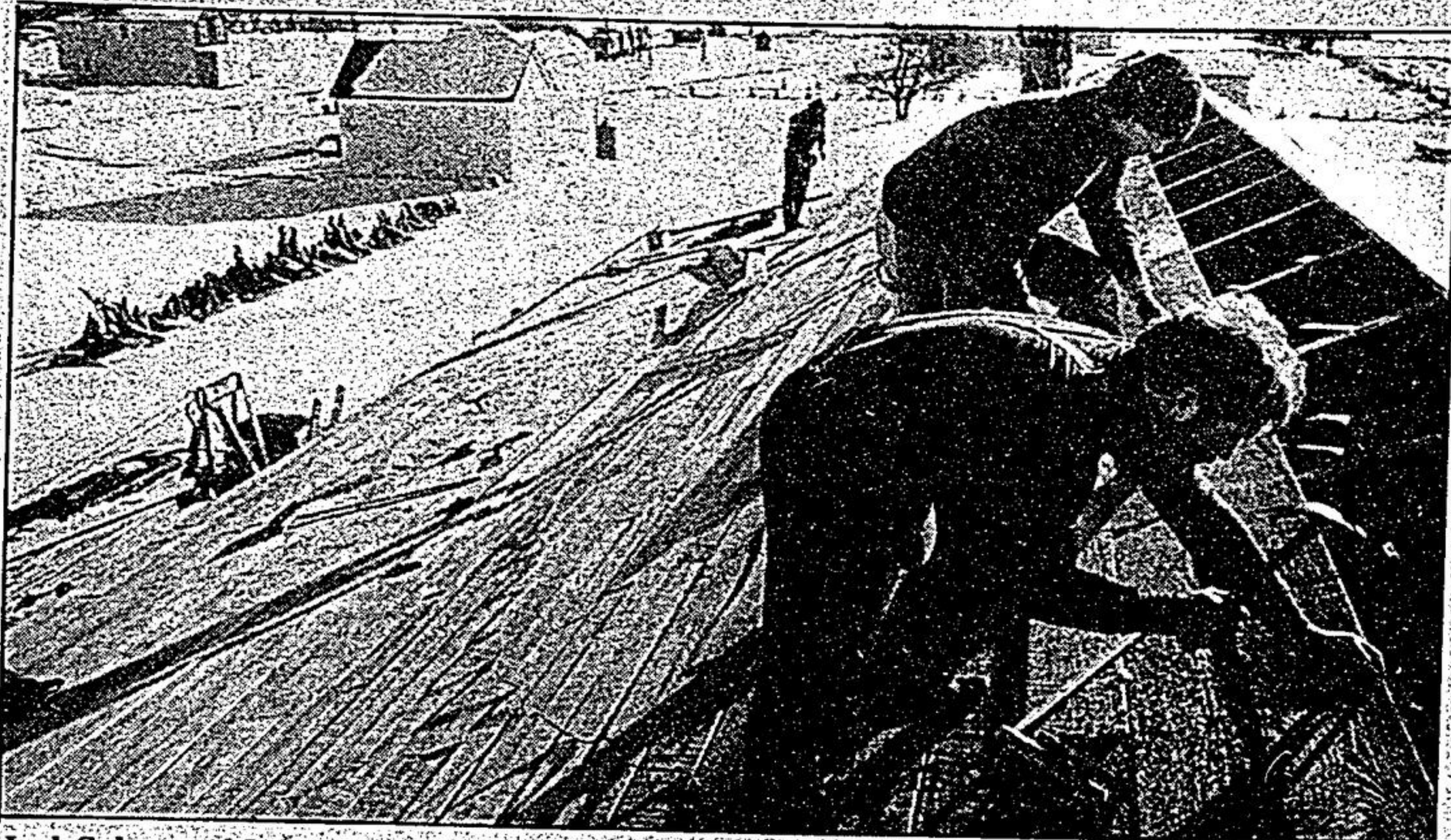
Jack Gubser and James Kennedy (front) put the last few boards on the roof.
