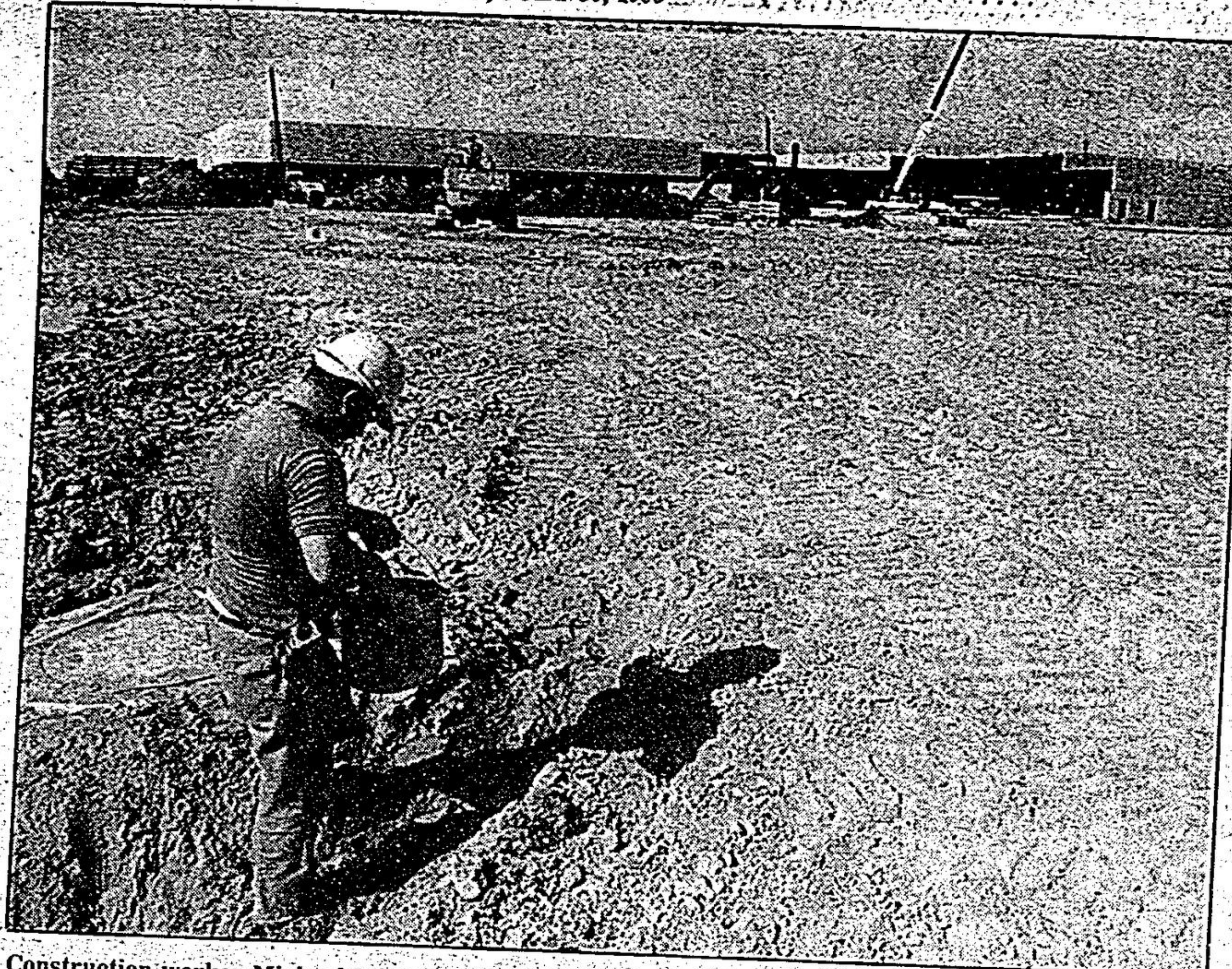
Construction worker Michael Malfora works on a catch basin as crews continue building Milliken's first covered shopping mall in the background. Officials expect the project to be completed by October. — Sjoerd Witteveen
