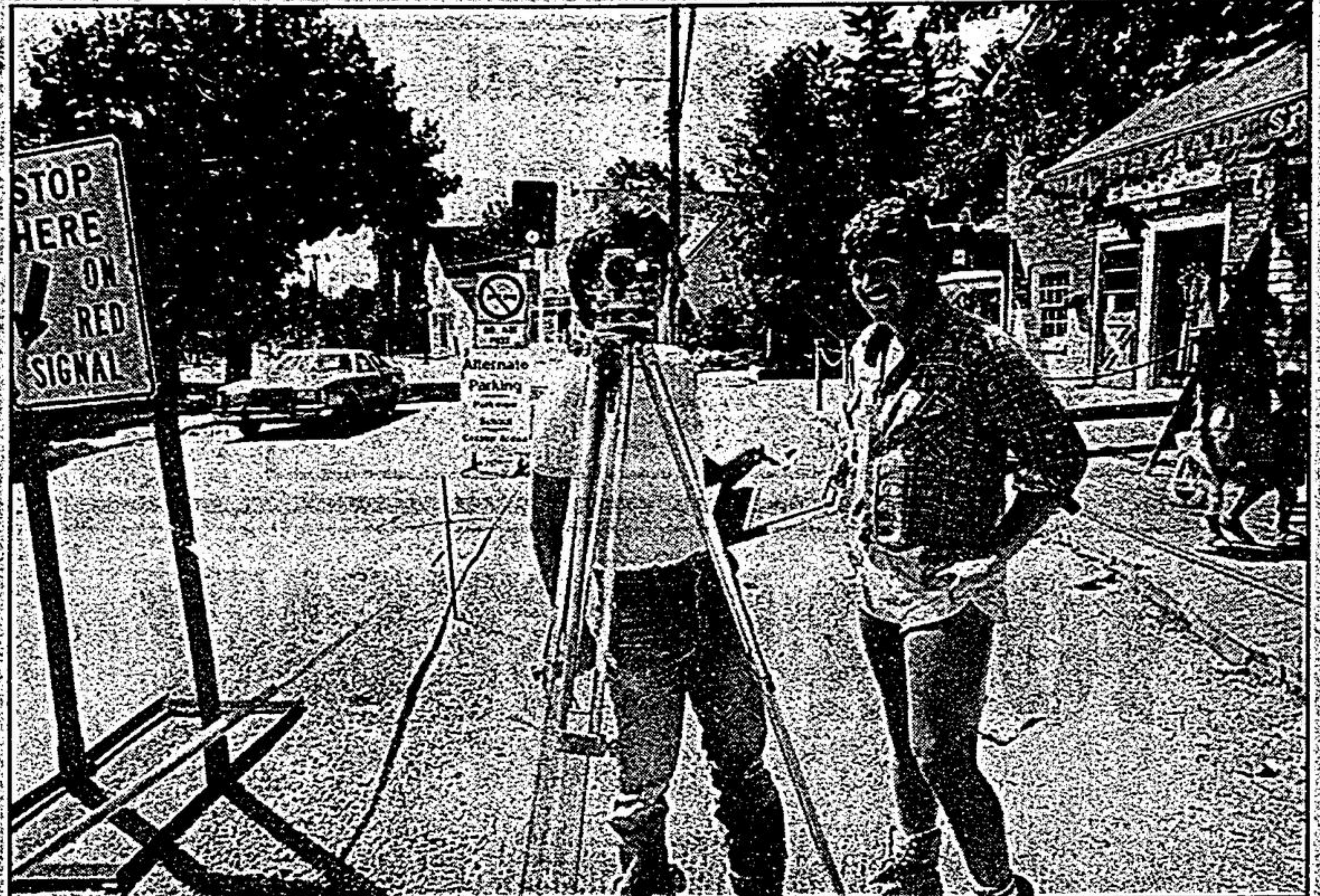
Surveyor Fred Watt checks the alignment while Dave Rendimonti looks on during Main St. construction in Unionville. Merchants seem resigned
