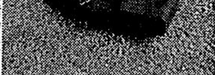
Rear heating ducts. Standard.
