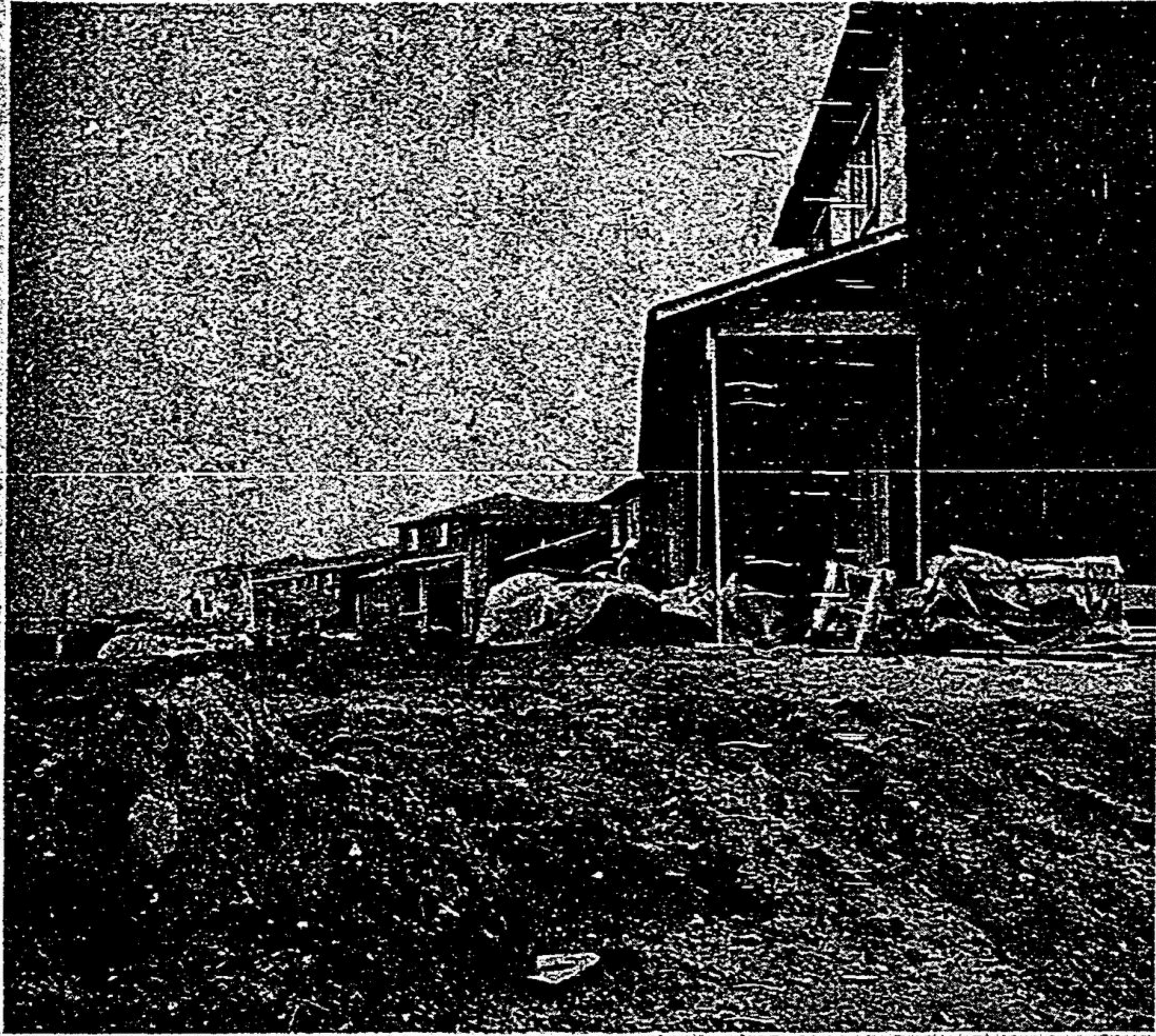
Northdown Homes project (also known as the Thicketwood subdivision) is progressing well. Here some of the model homes are under construction. The project will contain 130 homes built in two stages.
