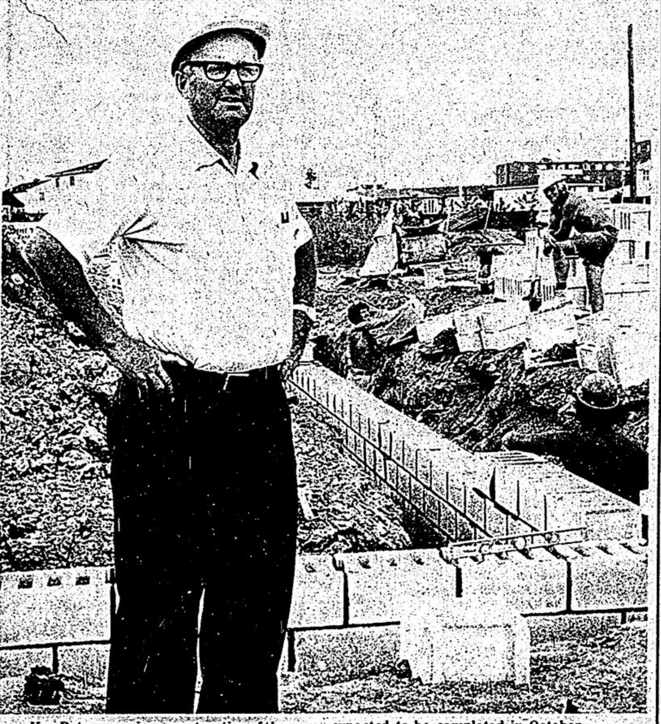
Ken Betz supervises construction of the new building to house Betz Pools Ltd. The building is expected to be completed in October. Ted Wilcox
