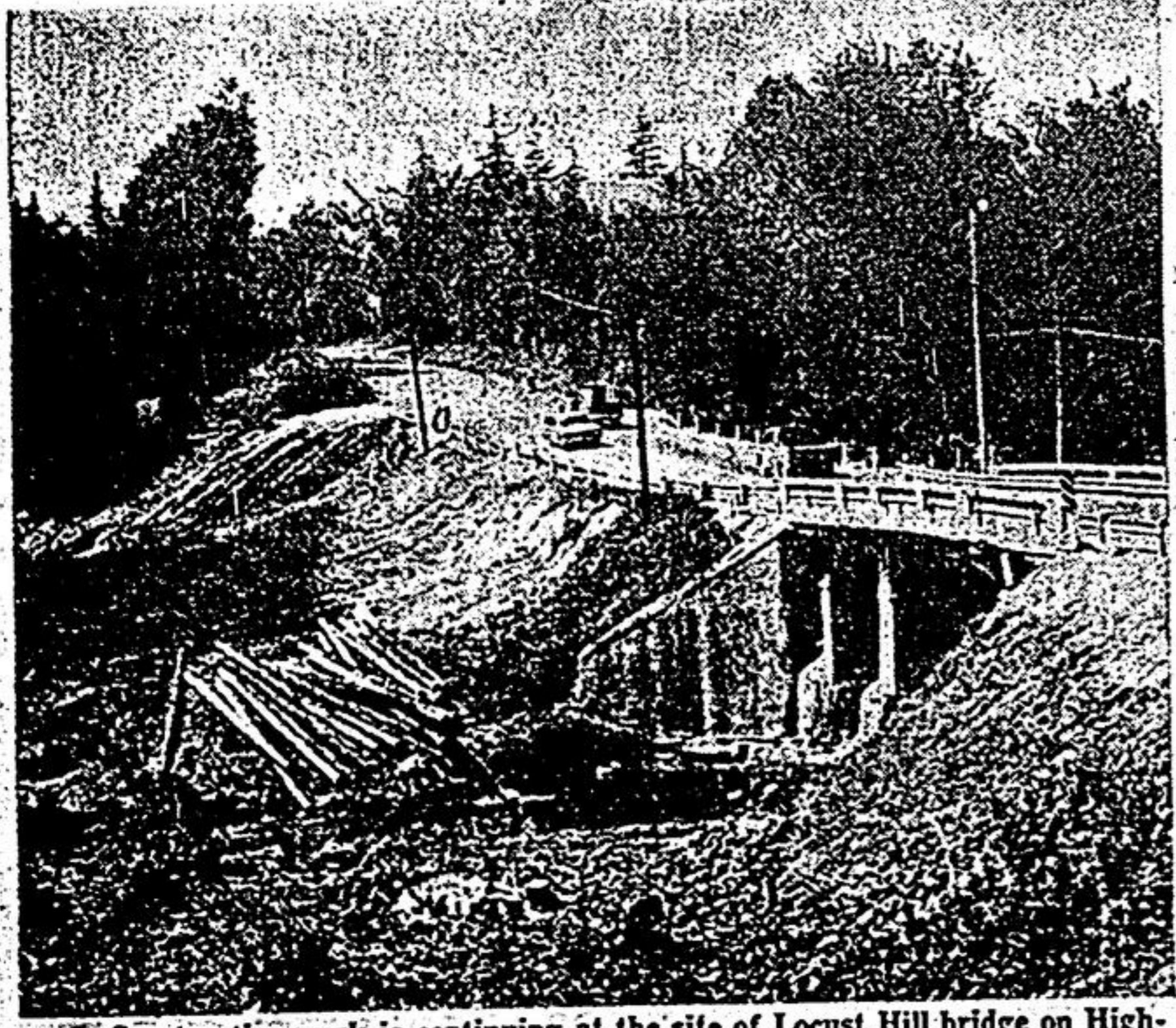
Construction work is continuing at the site of Locust Hill bridge on Highway No. 7. It has long been a bottleneck for traffic in the area. —Staff Photo.
