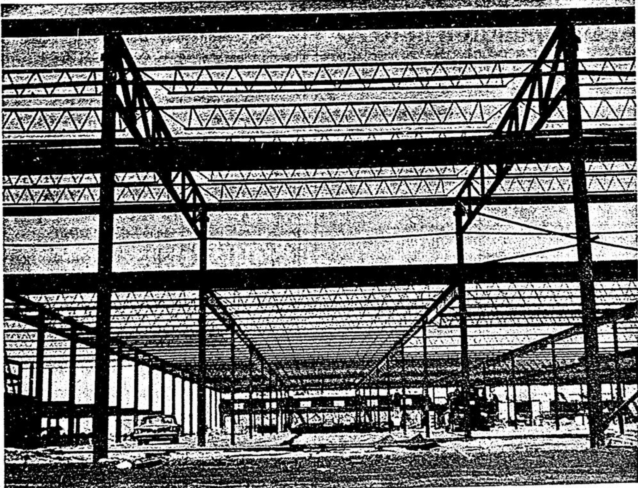
The "skeleton" steelwork of the new Amalgamated Electric Corporation plant and office building is rapidly taking shape in the Village of Markham. The factory, when completed, will cover 130,000 square feet of floor space and will be ready for occupancy by Fall. The site, west of the Chesapeake Ponds plant includes 10½ acres of land.
