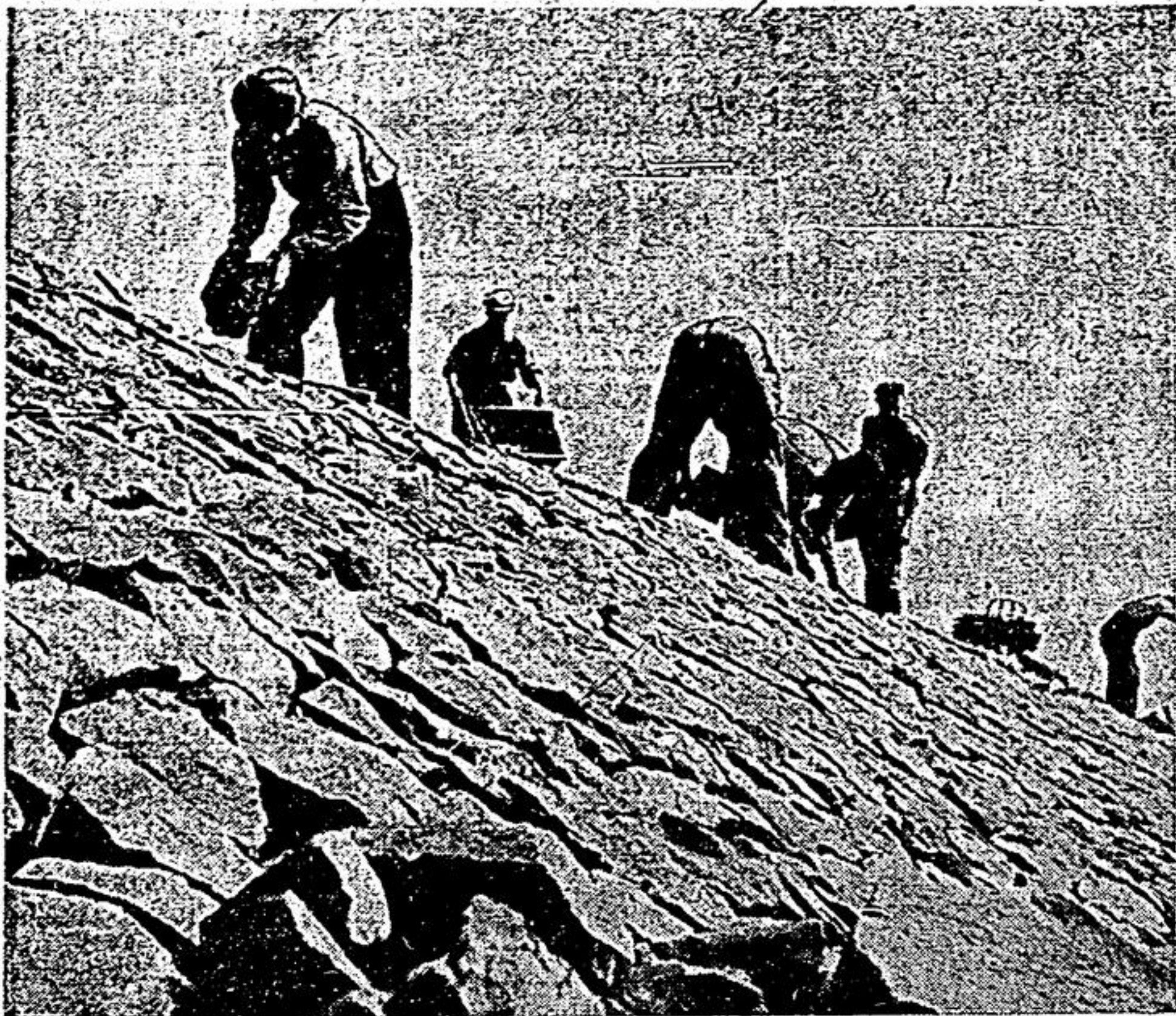
Workers strengthen foundations by setting blocks into place along a dike wall.
