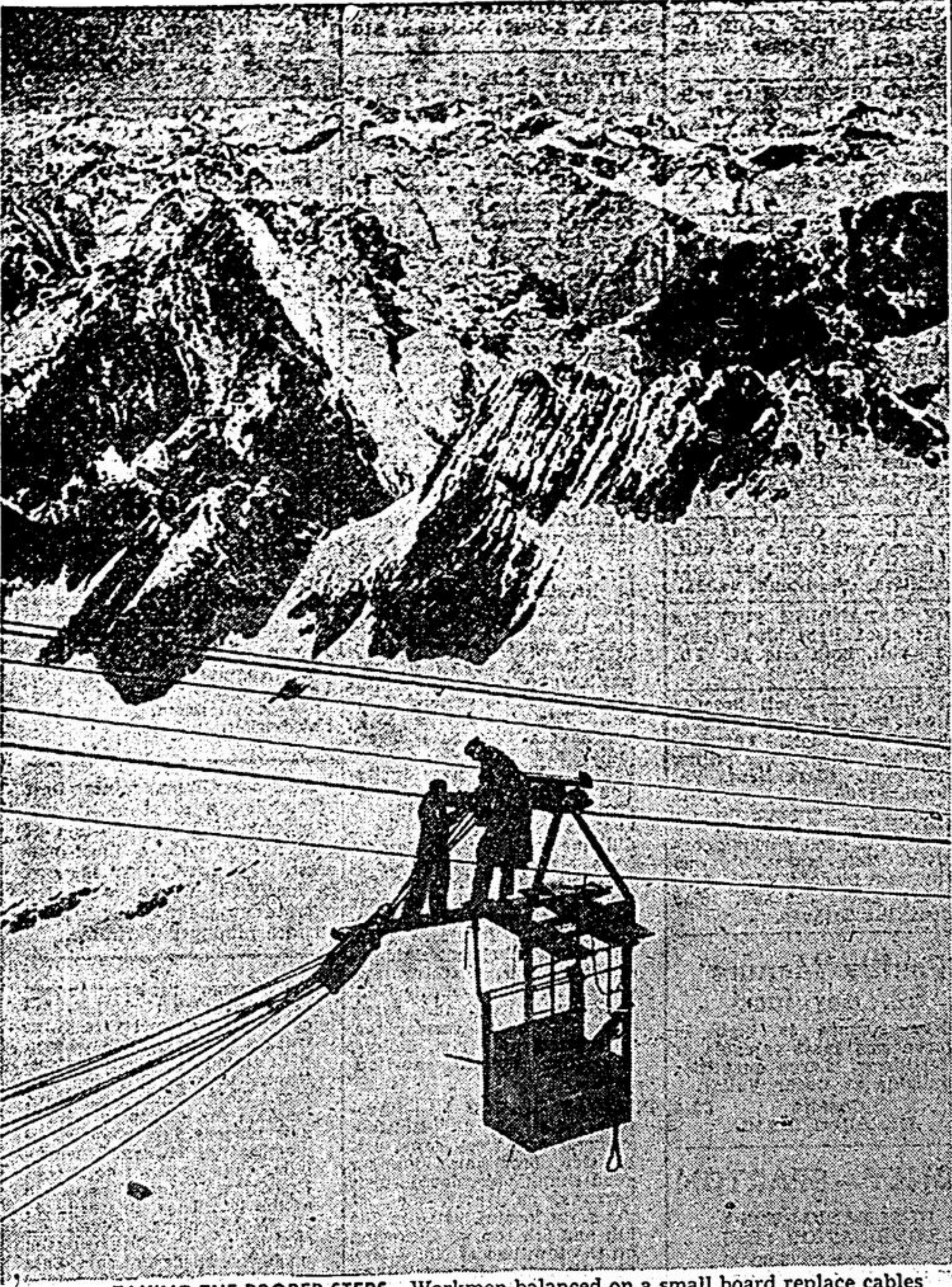
TAKING THE PROPER STEPS —Workmen balanced on a small board replace cables on the Zugspitz cable car high over snow-covered mountain ridges near Garmisch, Germany. The car connects a plateau with 9,720-foot-high mountain.
