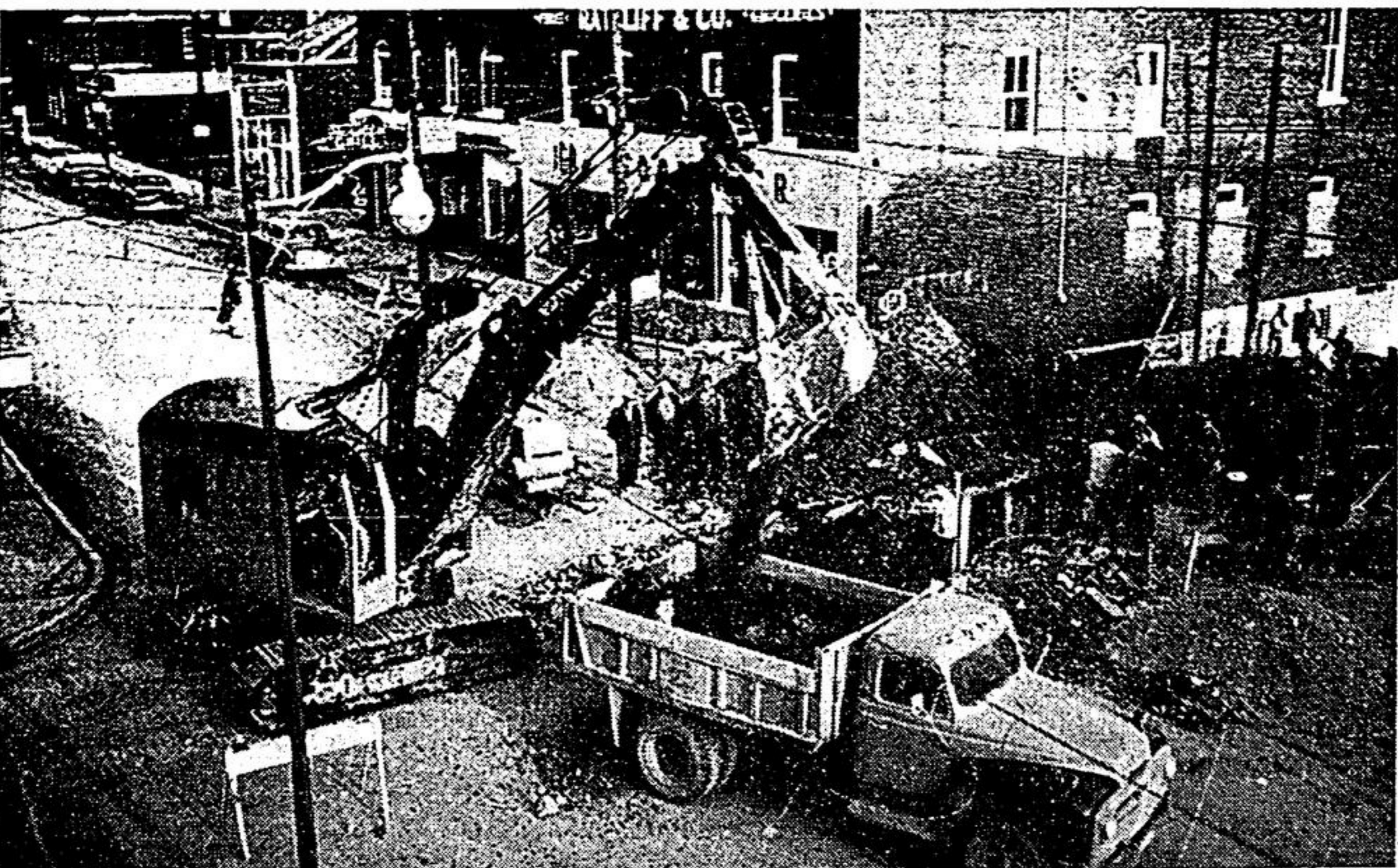
Seen from atop the news-paper office, one of the large power shovels is cutting across Main Street at the busy corner of Market Street, thence north on Mill Street.
