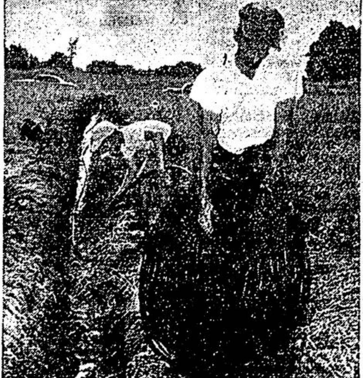
A PIPEDREAM COMES TRUE for the man on the land. The flexible plastic, C-I-L Polythene makes pipe-laying chores a cinch. All he needs are a rough trench, a saw for cutting pipe lengths and a screwdriver for tightening fittings. Flexible polythene bends around rocks, curves and corners.
