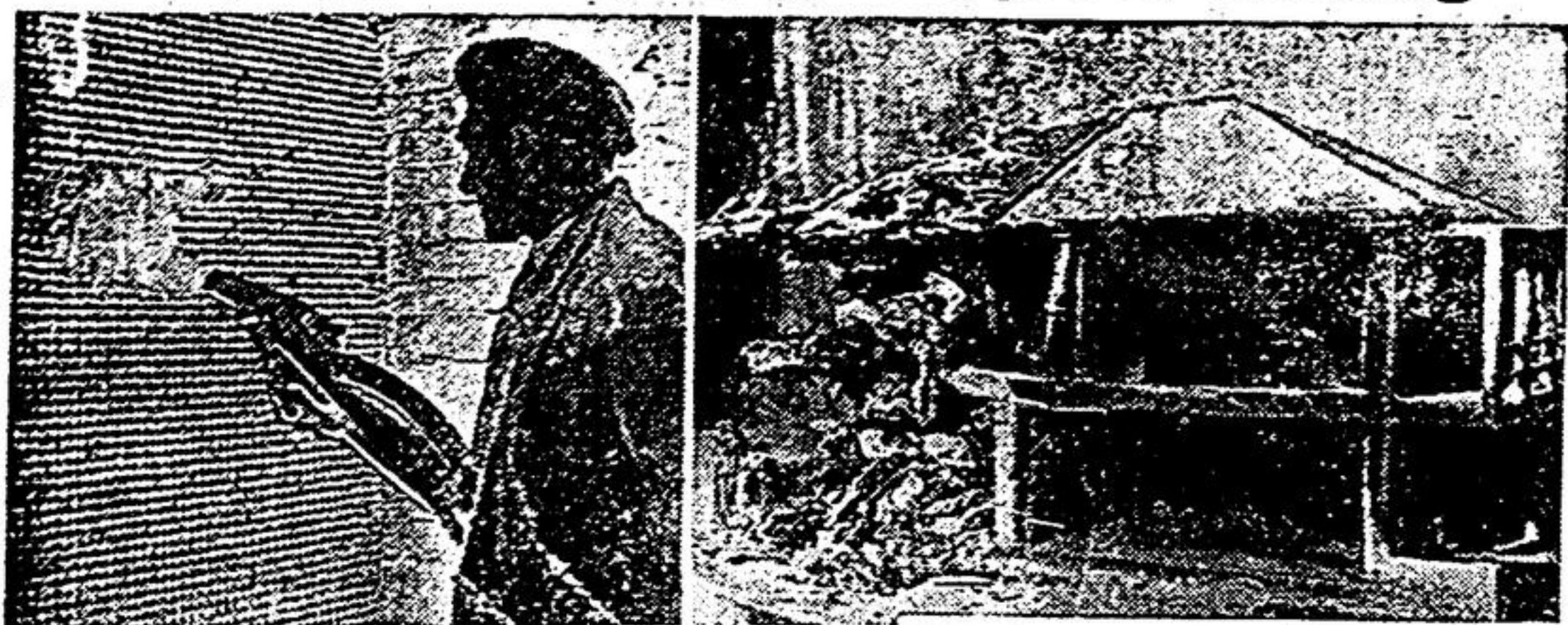
COMBS BLEW UP or damaged 4,500,000 British homes, so the British are now blowing up—with spray guns—houses to replace the loss. The walls of these new homes are wire frames sprayed, to a thickness of 8 inches if necessary, with a new material developed in Britain and named Pyroc. Fireproof and non-cracking, Pyroc sets hard in 50 minutes, takes nails or screws, and cuts with an everyday saw. Top left: It is sprayed on to the wire mesh. Bottom left: The mobile tank in which it is mixed and the sprayer (right) at work. Top right: Model house shows Pyroc's fireproof qualities. The collapsed part (left) had not been treated with the new material. By the end of this year Britain will have completed, since August, 1945, 750,000 new homes, housing, in all, about 3,000,000 people.
