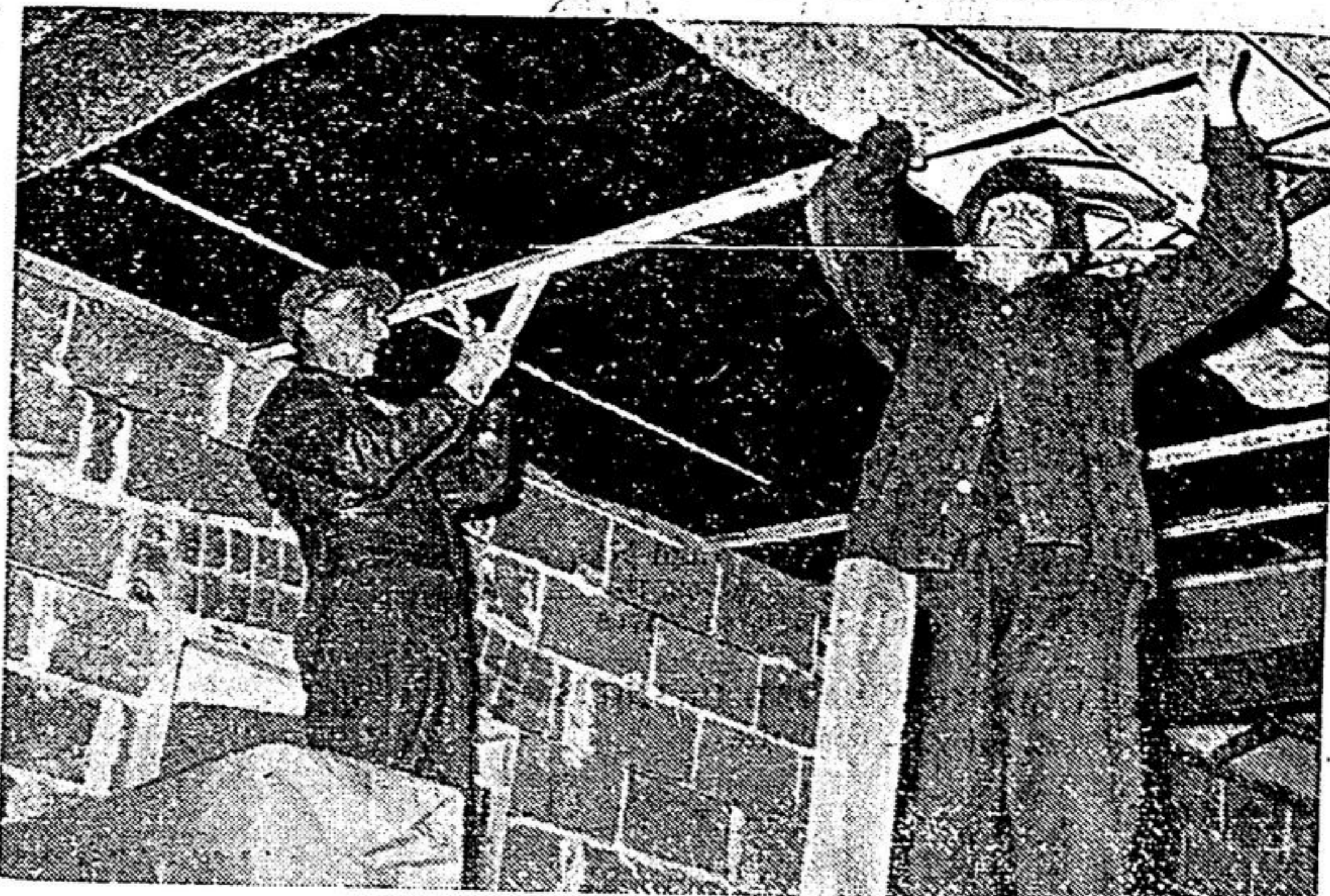
Interior of the new church will be finished by September 1, members' hope. Frank Herbert and W. A. Hiltz (left to right) are seen insulating the ceiling.
