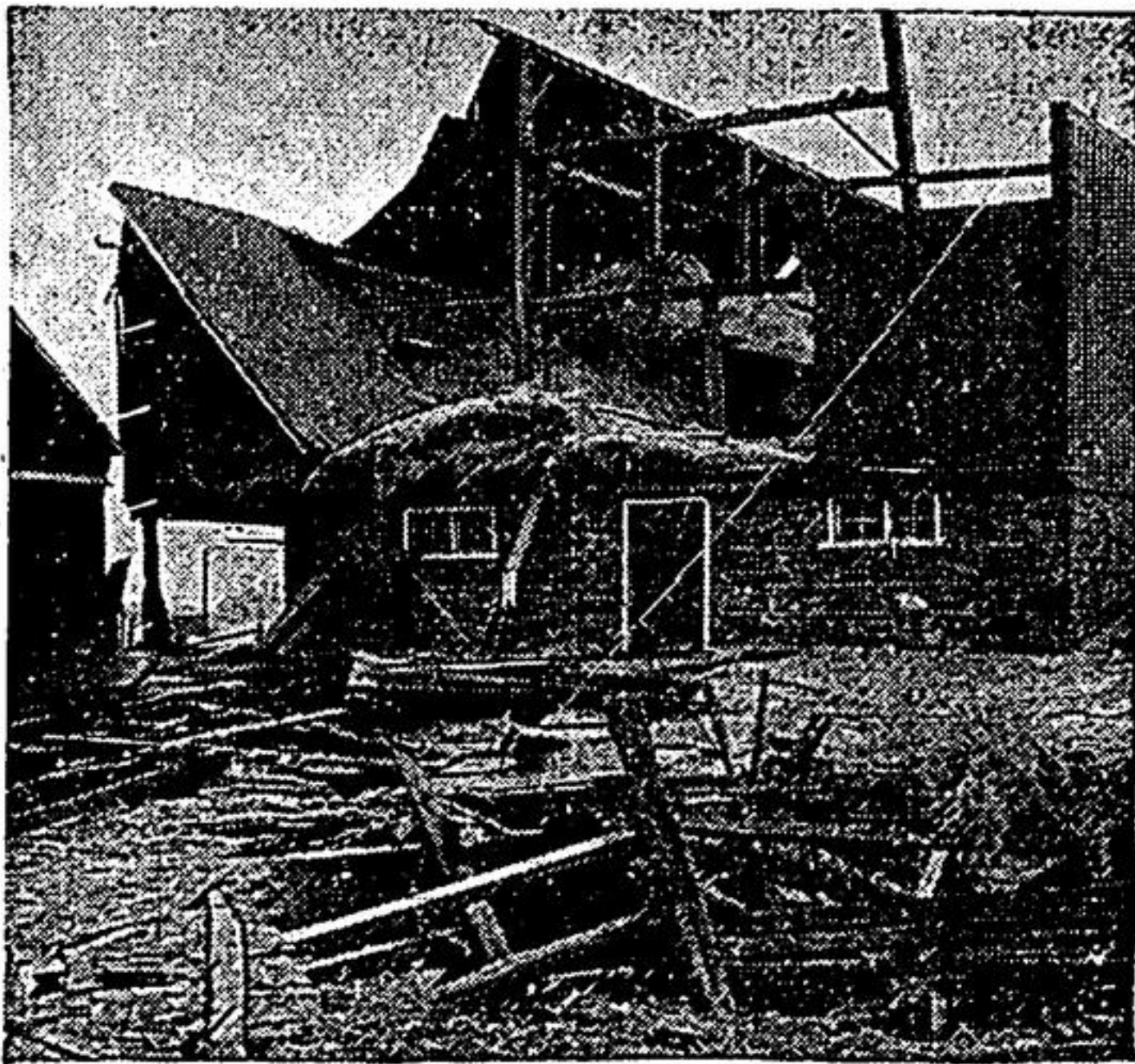
This barn is on the farm of Harvey Burkholder, No. 7 highways, almost due south of Stouffville, and shows how Sunday's storm played havoc with the sturdy structure. Other barns in Markham Township suffered a worse fate than the one shown here.
