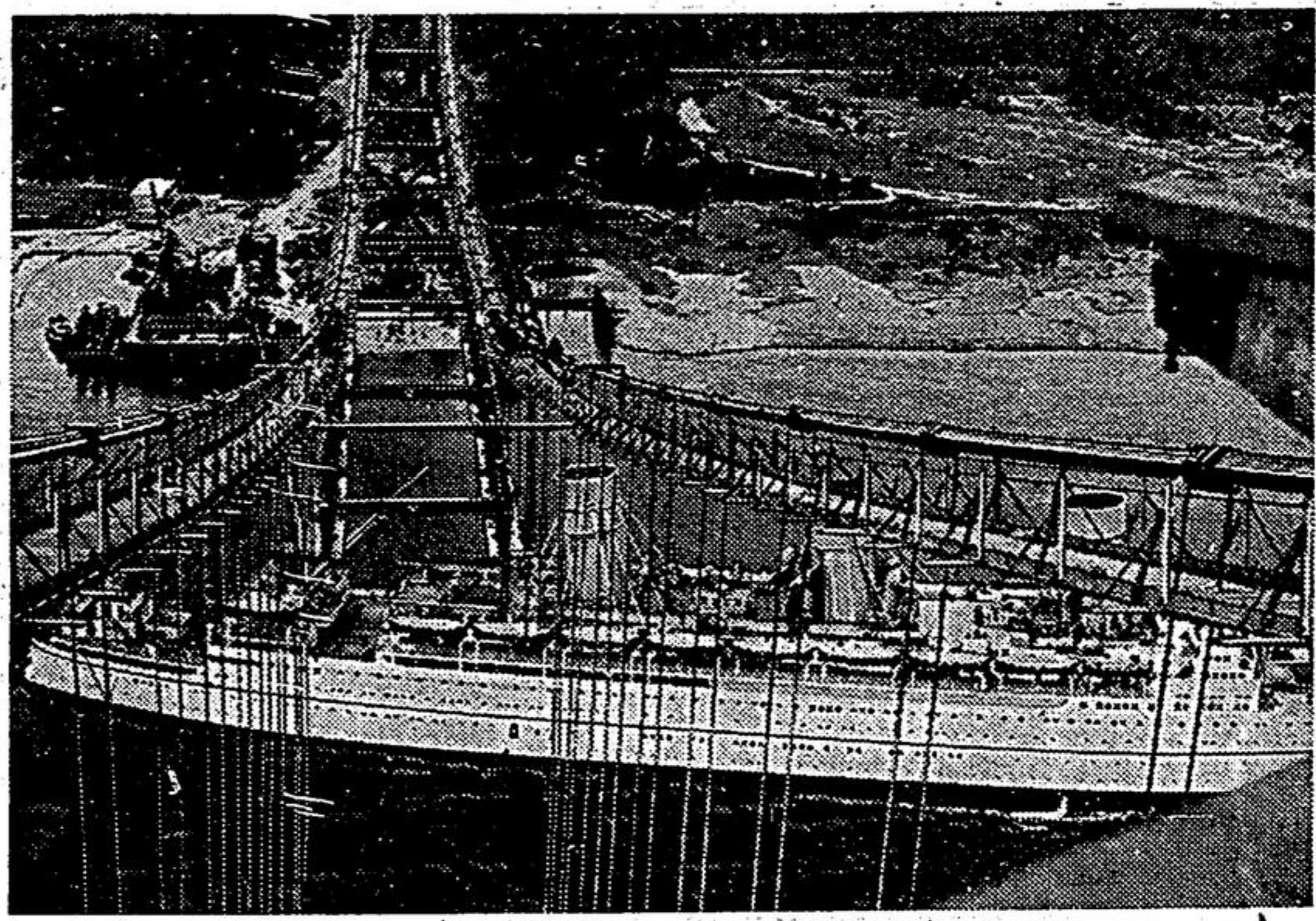
The Empress of Japan, Queen of the Pacific, passing under the splendid new bridge now under construction across the First Narrows, the entrance to Vancouver's landlocked harbor. The mainmast
