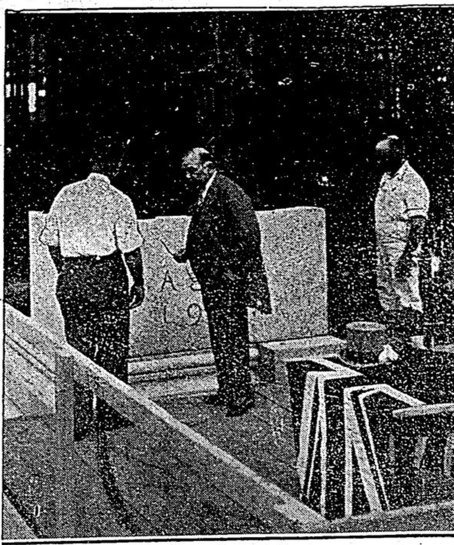
Rt. Hon. W. L. Mackenzie King is here seen, trowel in hand as he "well and truly" laid the corner-stone of the new Bank of Canada building in Ottawa. To the right is Graham F. Towers, Governor of the bank.
