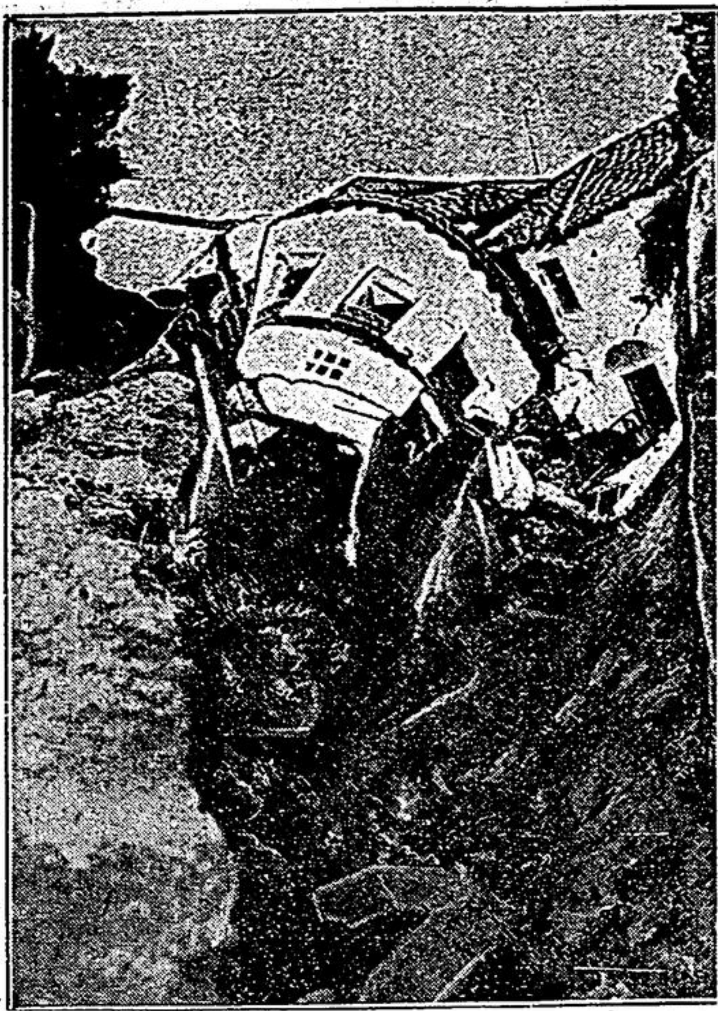
Close-up of the demolished home of Mayor Thomas Murphy of San Clemente, California, showing how it tumbled into a deep crack when the bluff on which it was built gave way.
