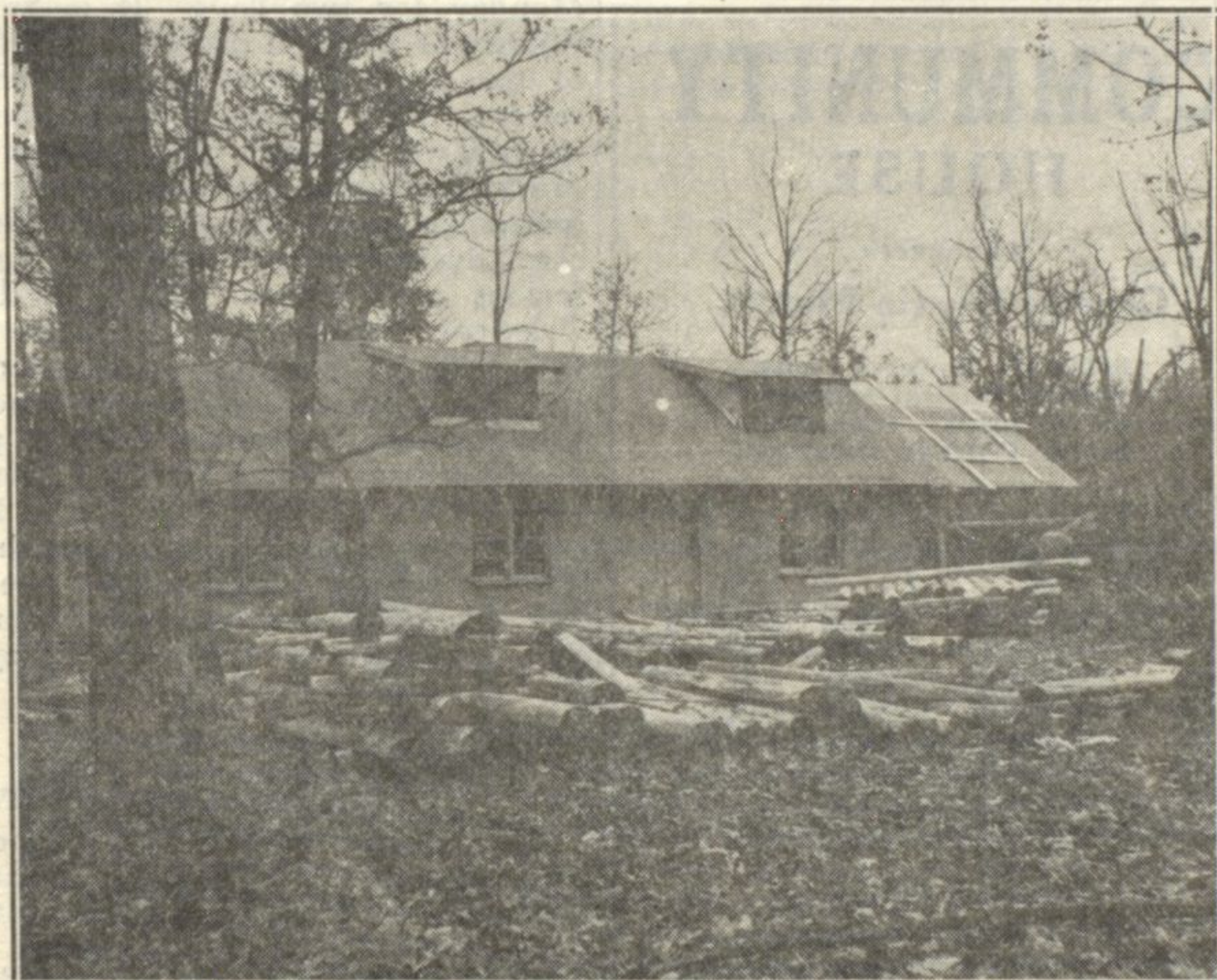
West View of Cabin—In the foreground are the logs shaped and prepared for facing the exterior of the cabin.
