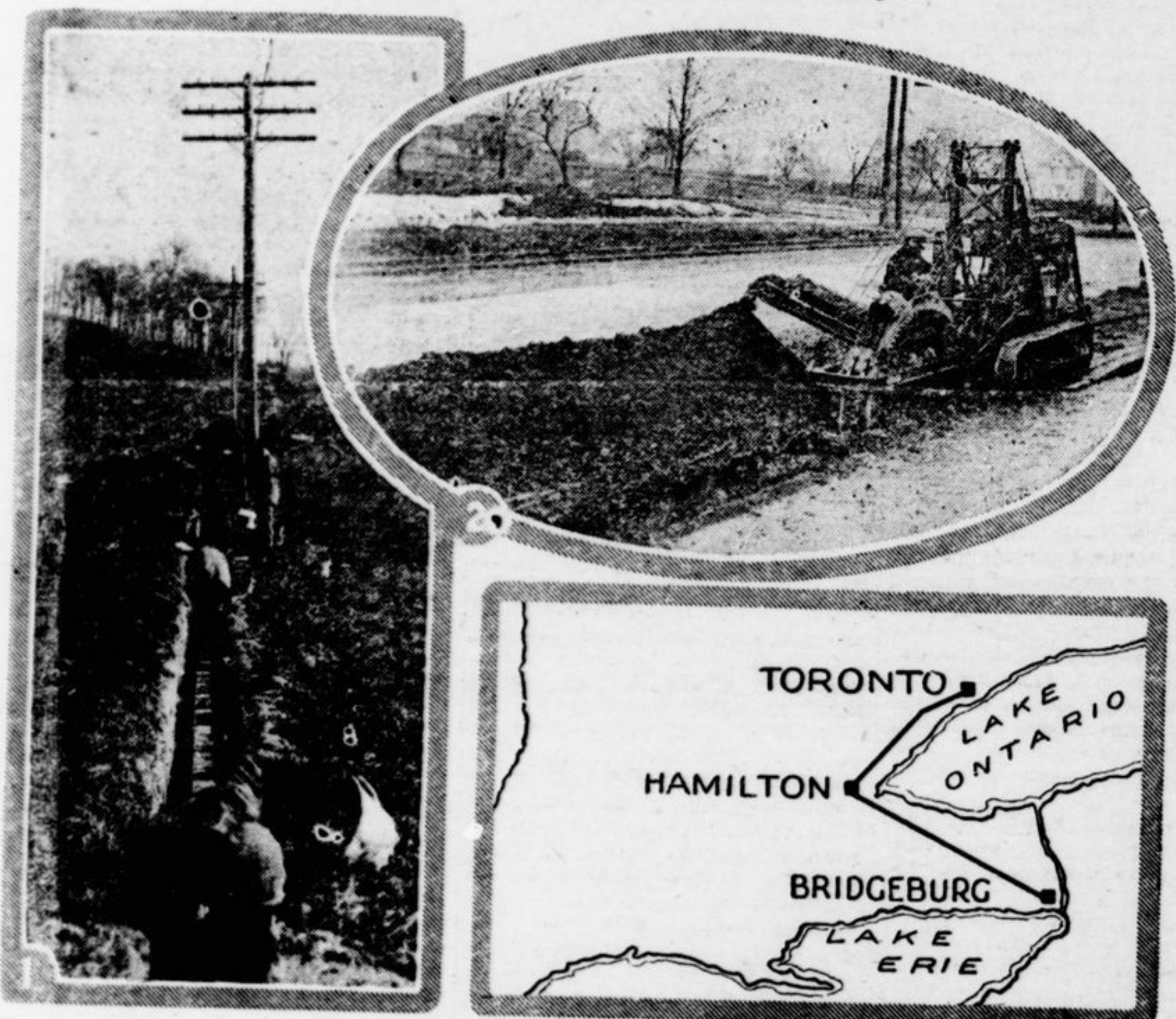
It was only a short time ago that science found a way of putting long distance telephone lines in cables. Already the first big job of erecting telephone cable (106 miles from Toronto to Buffalo) is nearing completion.
