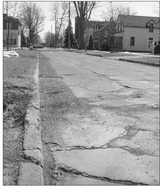
ROUGH ROAD – During budget talks Mar. 6, Essex Town Council recommended delaying the reconstruction of Alice Street in Essex, pictured above, a $235,000 project originally scheduled for 2007, under the town's 10-year road plan.
