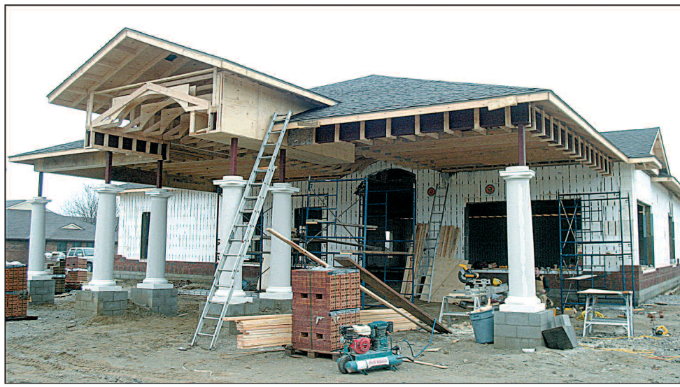
For a better community - Mild weather has helped speed construction of the Harrow Family Medical Centre, located just off Erie Street South in Harrow. The clinic is expected to open in May 2007.
