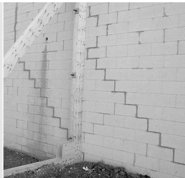
Wooden planks were installed outside Essex Memorial Arena in November 2005 to secure walls that were cracking. The problem was listed in a report conducted by a Windsor engineering company in April 2005.
