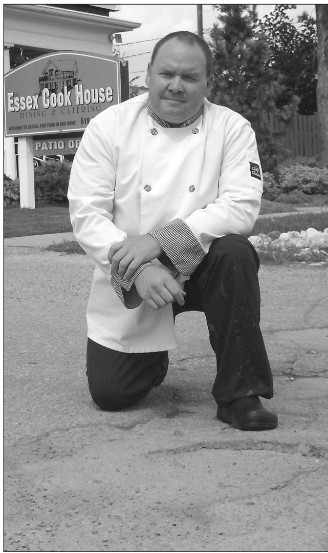
Essex Cookhouse owner Larry Girard kneels in front of one of many potholes lining Laird Avenue between Alice and Talbot streets. Town Council recently approved a 10-year, $21.5 million plan to pave 80 kilometres of roads in the municipality.
