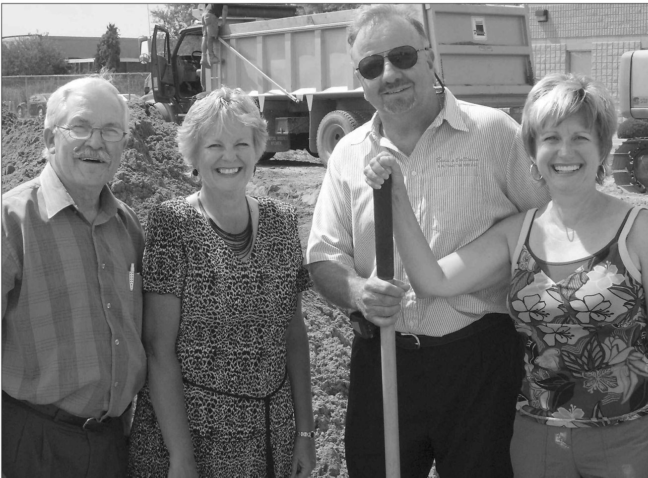
CONSTRUCTING A CAR WASH – Essex Mayor Ron McDermott, left, Dannie Quinlan, account manager for Woodslee Credit Union and Roger and Rita Beaulieu of Beau's Collision and Auto Service, break ground at the future site of a fully automated touchless carwash. The Beaulieu's are expecting to open the carwash in early November, which will offer six self-serve bay stations, a well-lit vending area, two vacuum stations and a water refill station. It will be open 24 hours a day and monitored by security cameras. Woodslee Credit Union is financing the project with construction by Marcovecchio Construction.
