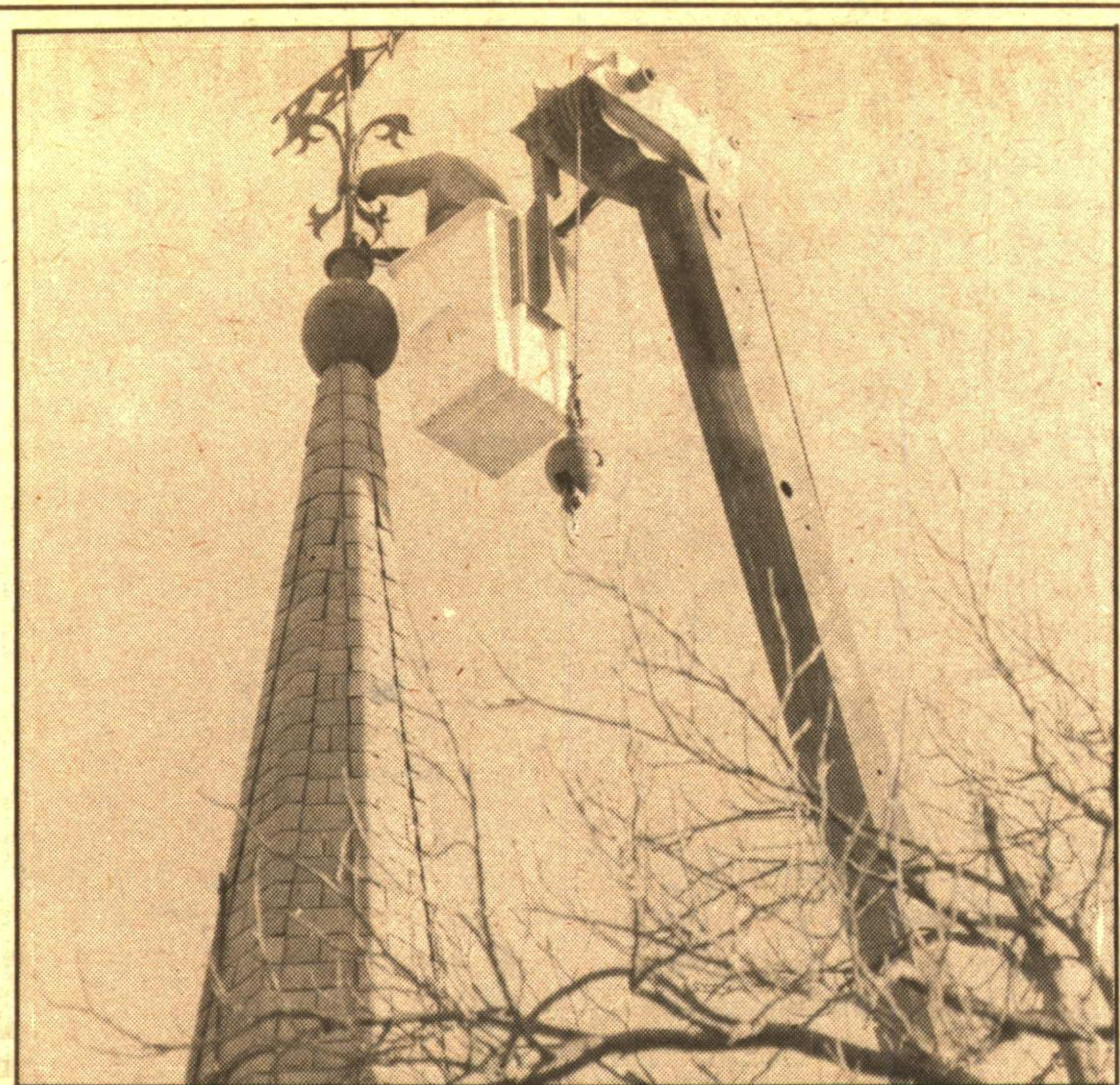
The weather vein atop the steeple of the old church which now houses part of the Georgetown library was leaning more than usual after a strong wind storm last month. So Cultural Centre Manager Hank Huhtanen decided to call H. Oversby Ltd., RR4 Georgetown, to straighten things out.
