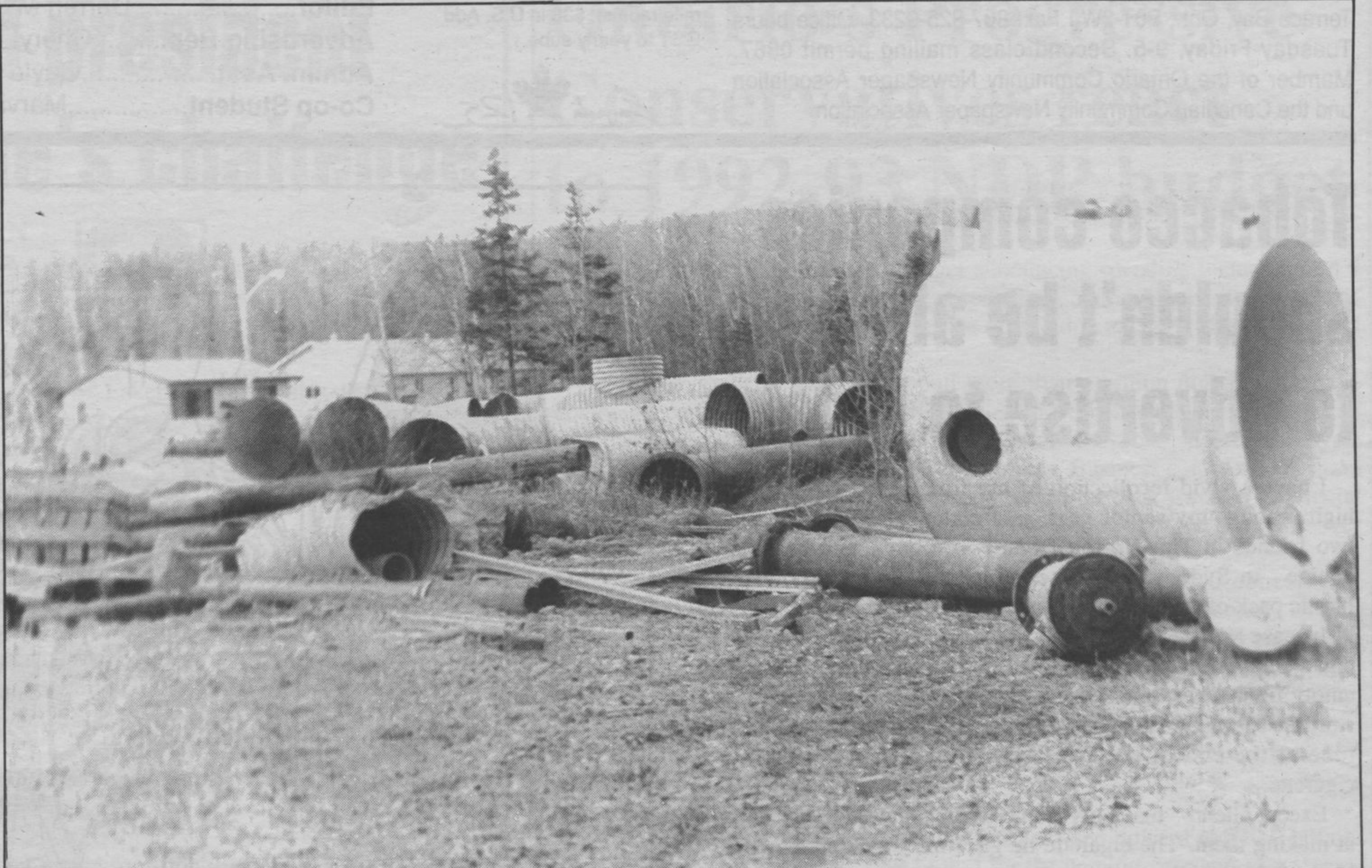
Some Peary Street parents say the culverts are a hazard to kids.
