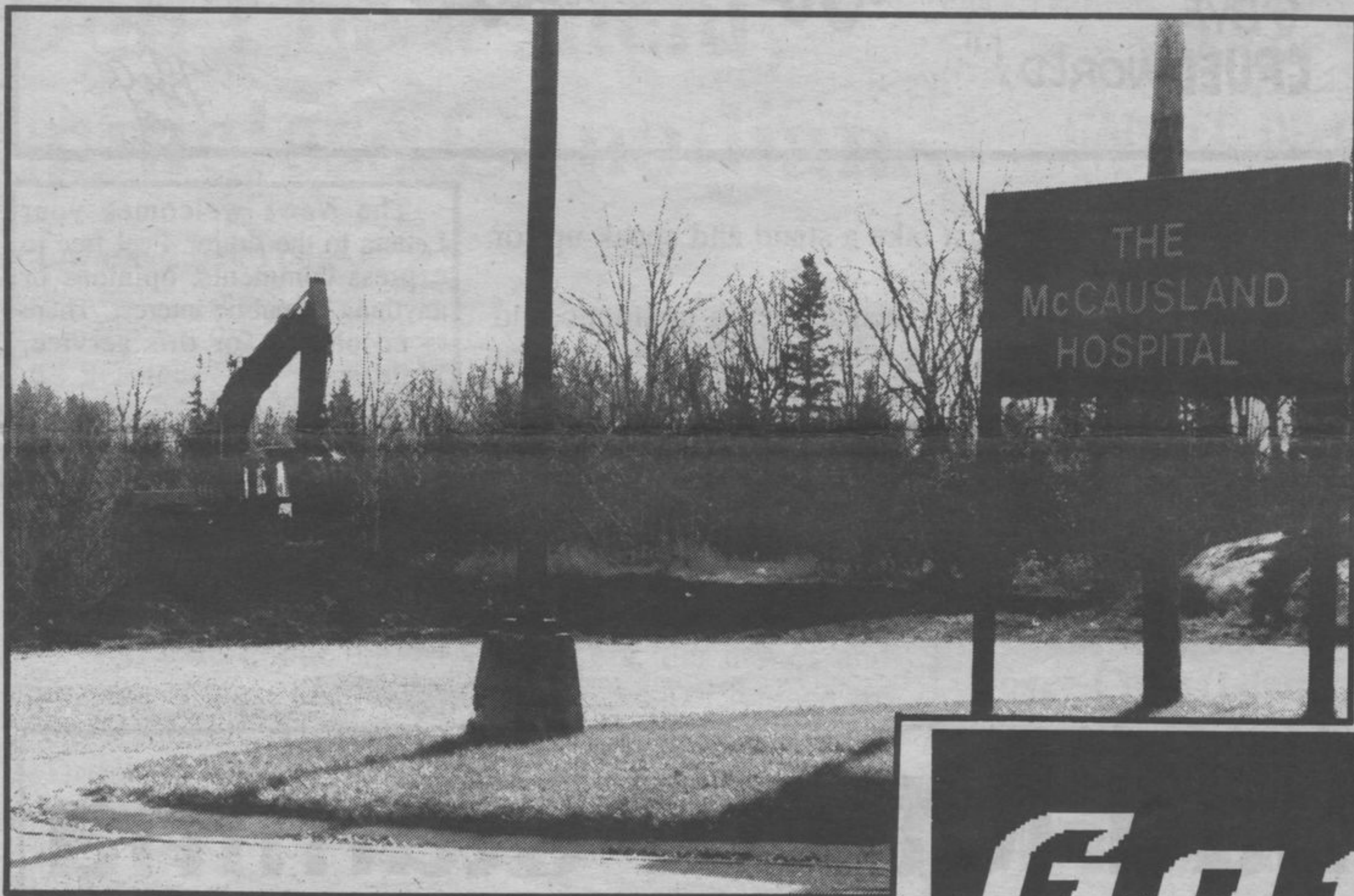
Ground work was started last week on what will be the new ambulance garage for McCausland Hospital. Curtis Desrosiers Construction Ltd. is carrying out the work. Photo by Dave Chmara
