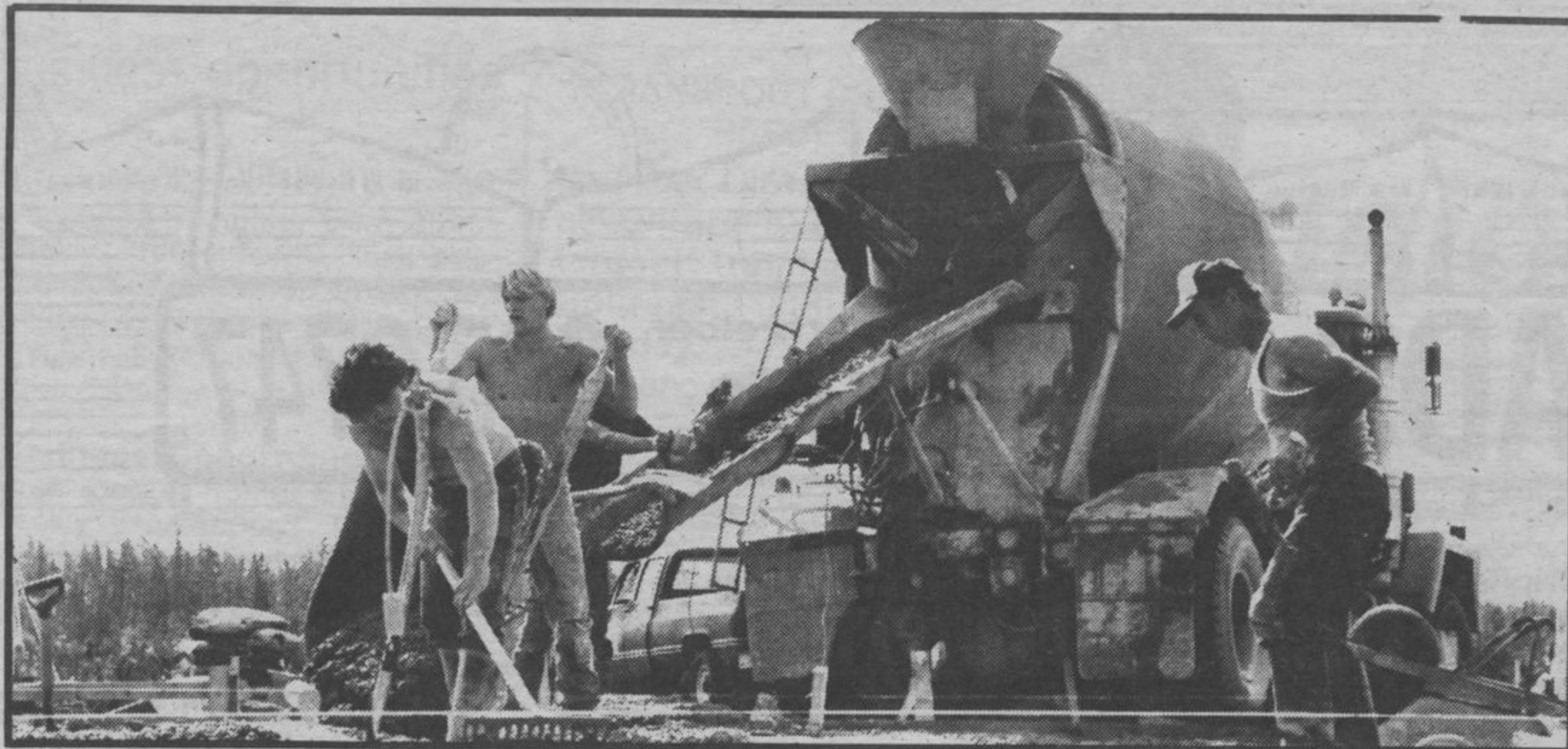
Tikal Ltd., based in Kakabeka Falls, is constructing the new airport maintenance garage which will be used to house the airport snowblower and other equipment. Photo by Dave Chmara
