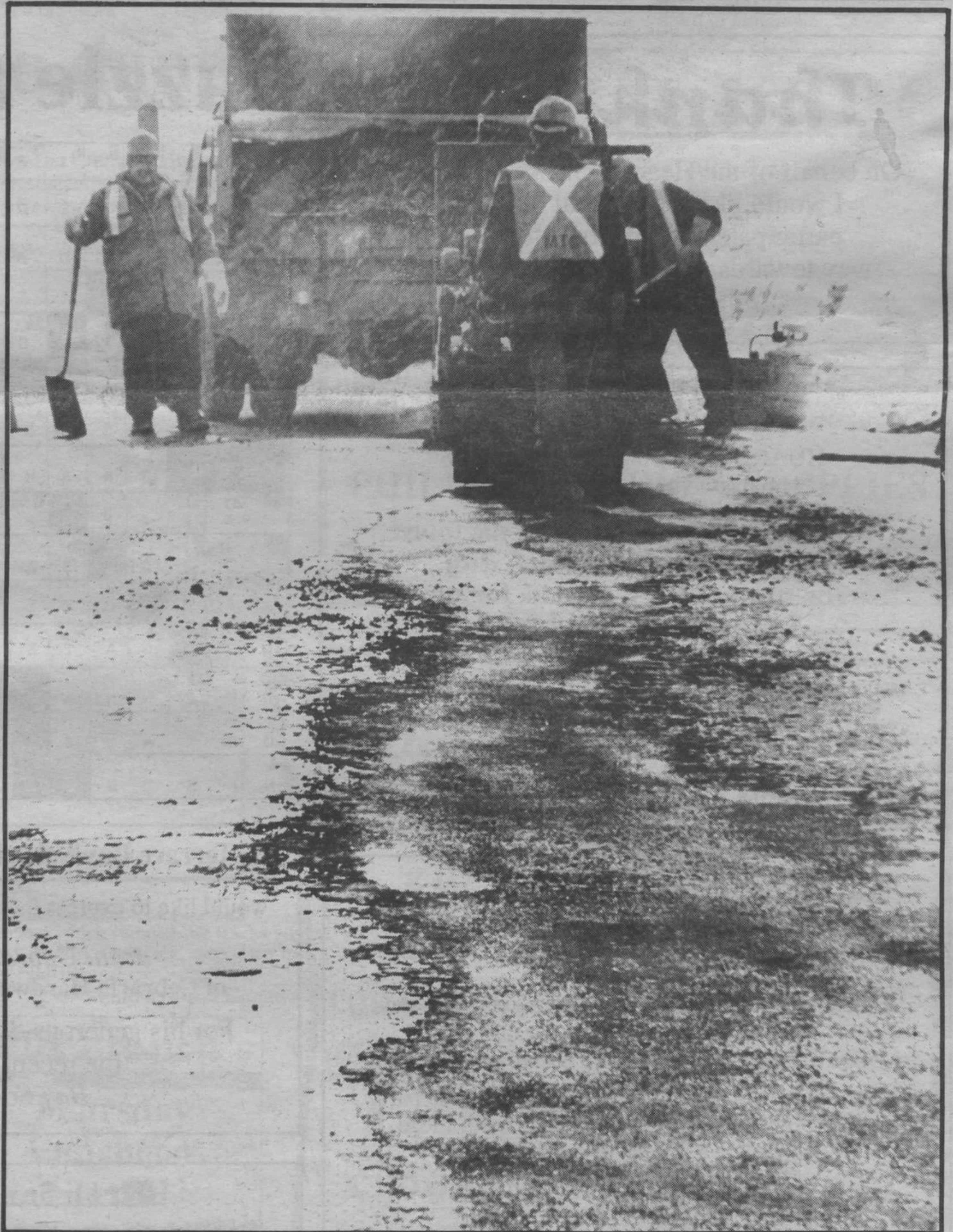
Ministry of Transportation crews work on a patch of road just west of the overpass which is east of Schreiber. It was less than two weeks ago that Terrace Bay and Schreiber town councils met with officials from the Ministry of Transportation to discuss problems with Highway 17 in this area. The severe bumps on this stretch of road were of prime concern to councils as is the snow plowing.
