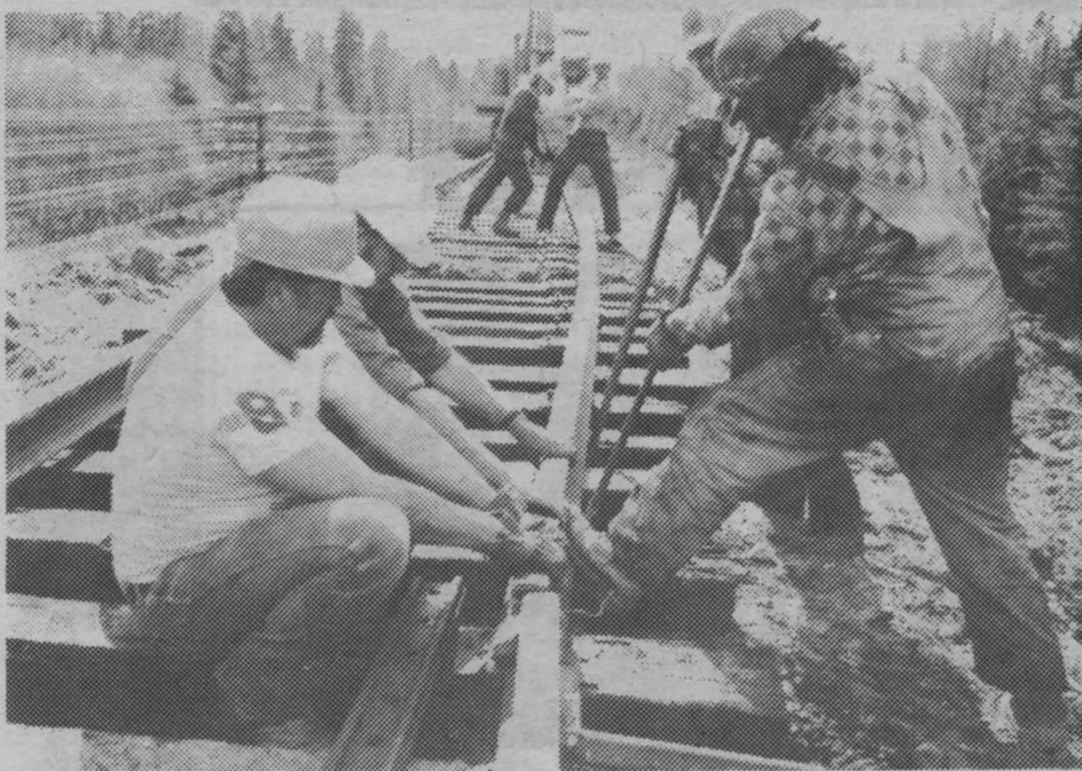
Making it fit: Section gangs under foremen Ken Michano and Robert Rasmussen struggle with pry bars to fit in a section of rail after a new culvert was installed on the division. Also assisting is Terrace Bay's own Dave Spear.
