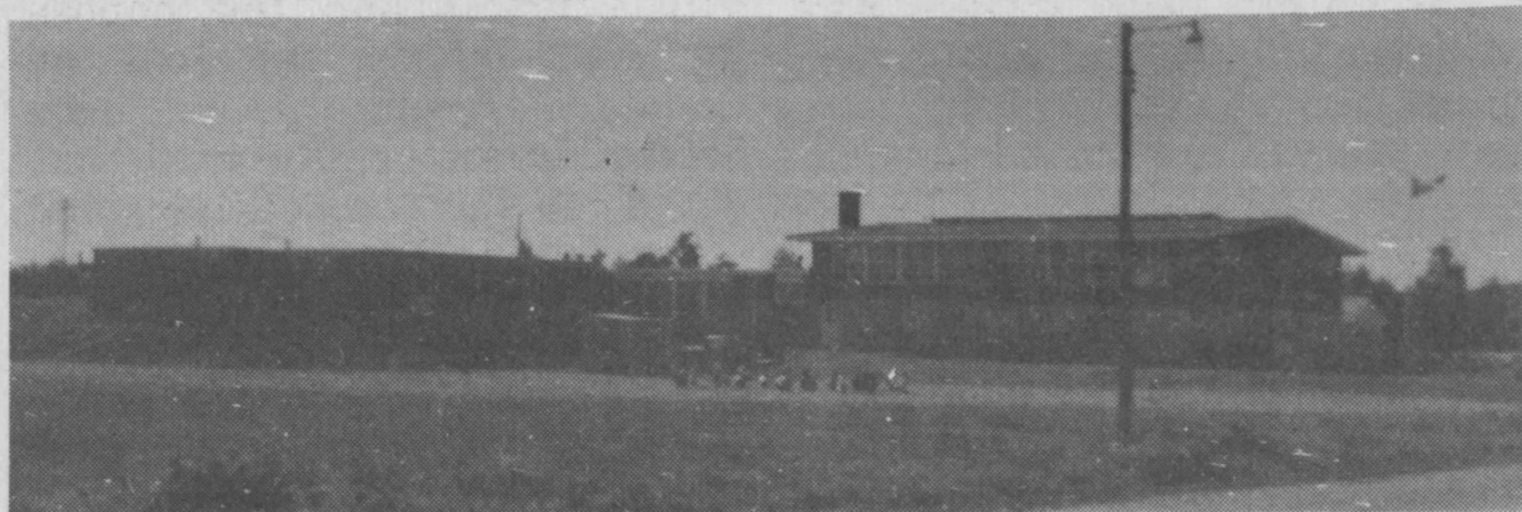
The $70,000 addition (two classrooms) being built by Cebrario & Sons to Holy Angels School. Photo by Inez McCuaig
