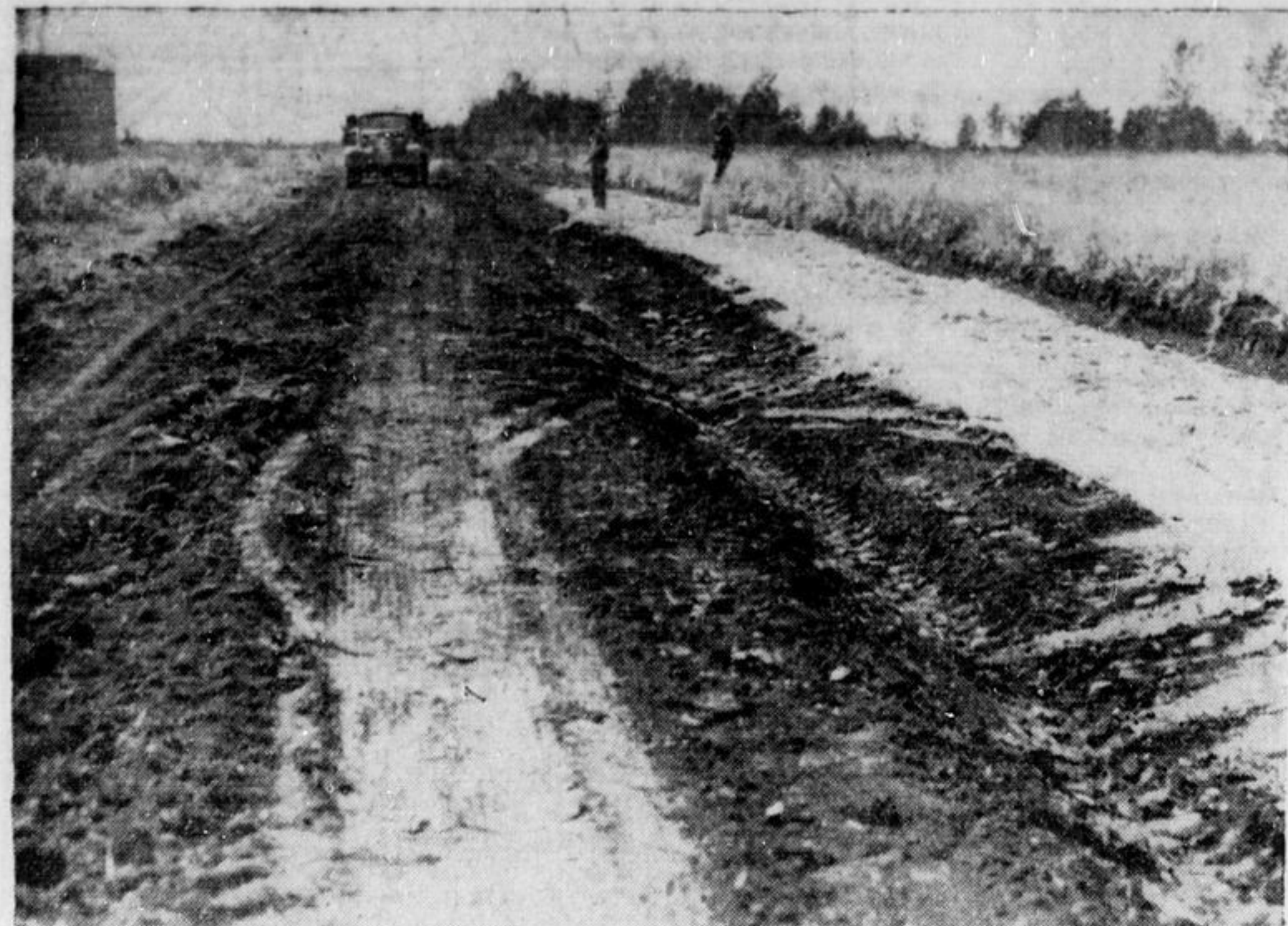
First move toward the opening up of Timmins' newest townsite, Westmount, in the northwest section of the town, began this week with work on a new road through the area by the Mascioli Construction Company.
