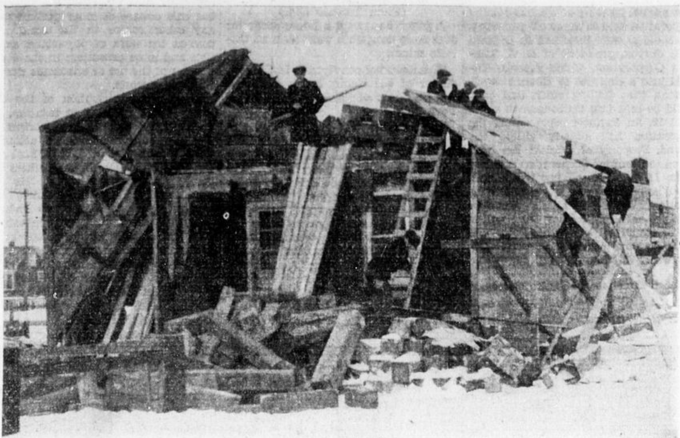
The above photograph shows what was left of a house seen at the left of the photo. One workman had his leg broken and another received a lacerated hand when they were caught under the falling roof.
