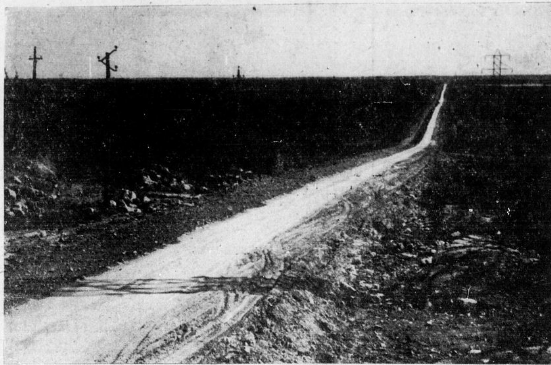
Work is progressing on the highway between South Porcupine and Schumacher. Last week-end the work of laying the cement was completed from near where the road turns into the Conlaum to the weigh scales at South Porcupine. With good weather it should not take long to finish the highway between Schumacher and South Porcupine and in a few weeks the highway should be open from Timmins to South Porcupine. The picture shows a stretch of the new highway on the Rae Hill. (Advance Photo and Engraving)
