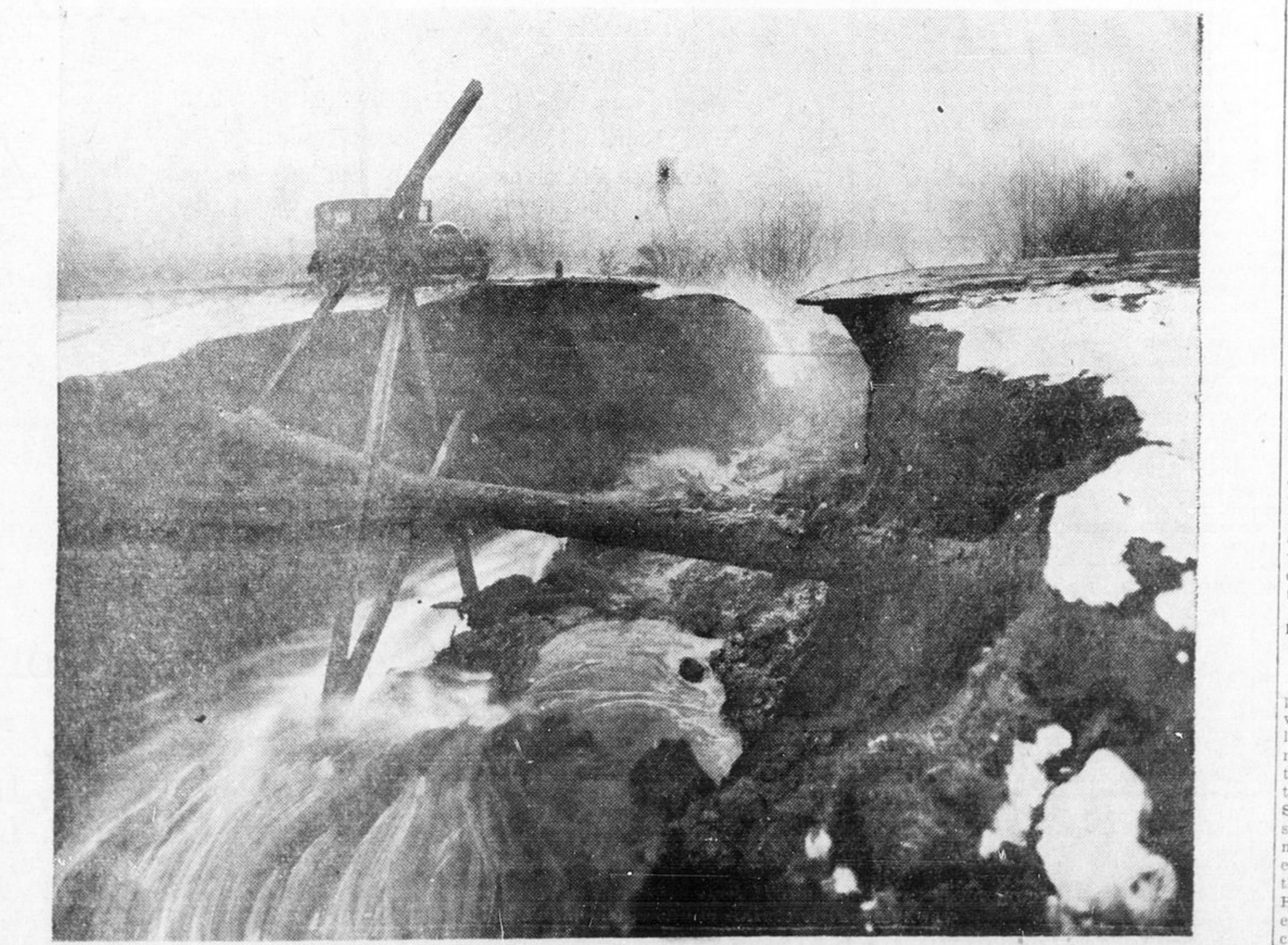
The power of the Valley flood is shown by this washout on the north road, Burquitlam. In the foreground is a broken watermain. The parked automobile is on the surface of the highway.
