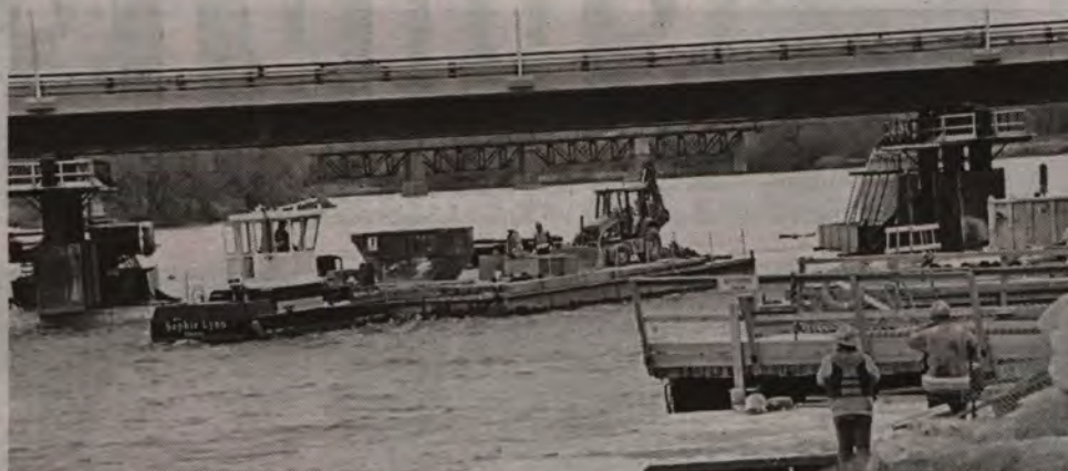
Work on the Cayuga bridge has come to a stop after the MTO failed to consult with Six Nations. (Photos by Jim C Powless)
