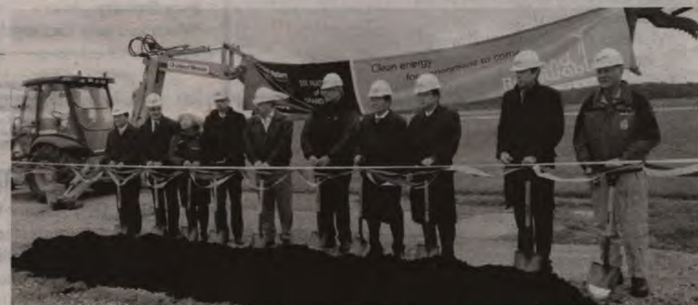
The massive Samsung project got underway with the cutting of a ribbon and ceremonial shovelling of earth. Then elected chief Bill Montour participated.
