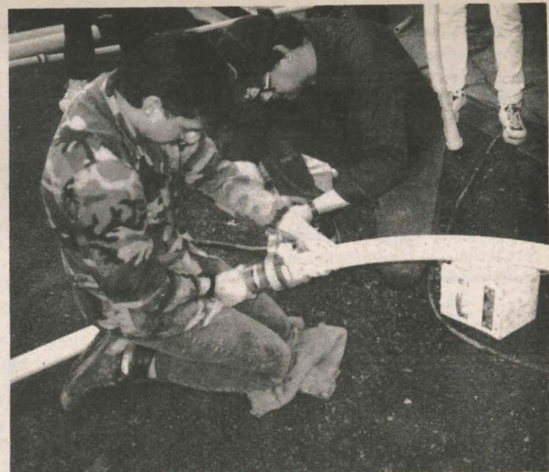
Curtis E. Hill and John VanEvery working on some of the buried pipeline used in the SN Natural Gas Company during the training and construction phase of the project.
