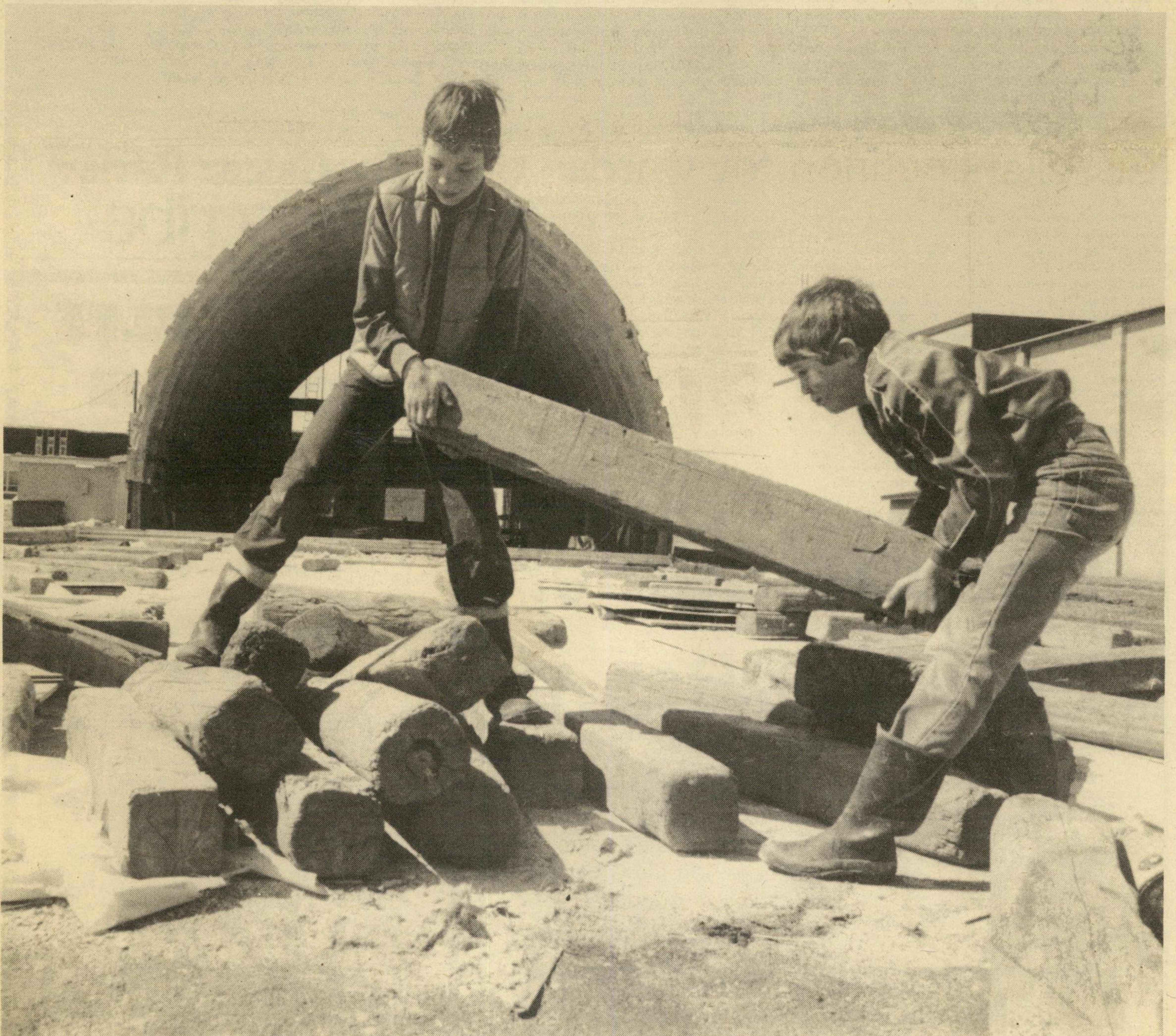
The Village of Metcalfe is to get a new curling rink, but first the old one had to be torn down. Chris McLaren and Warren Larry decided to help a hand with
