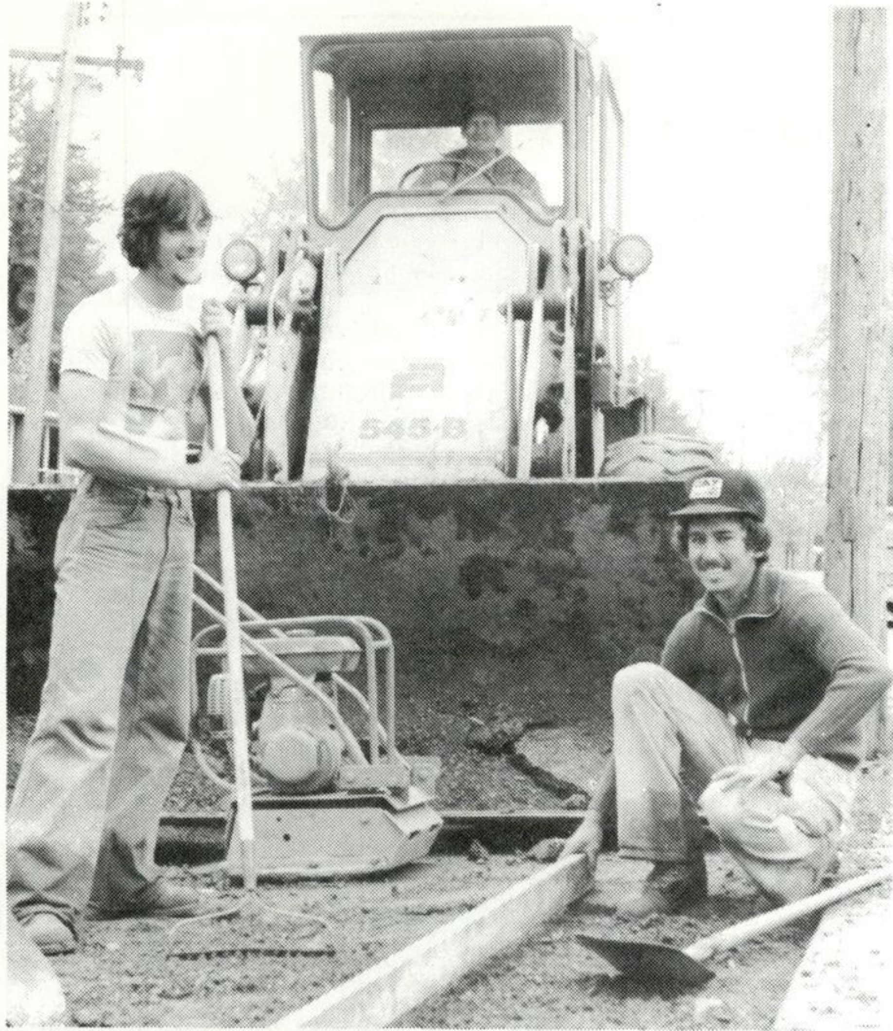
The smiles on these workers faces reflect the happiness of local residents as the final stages of paving are completed in Russell Village.
