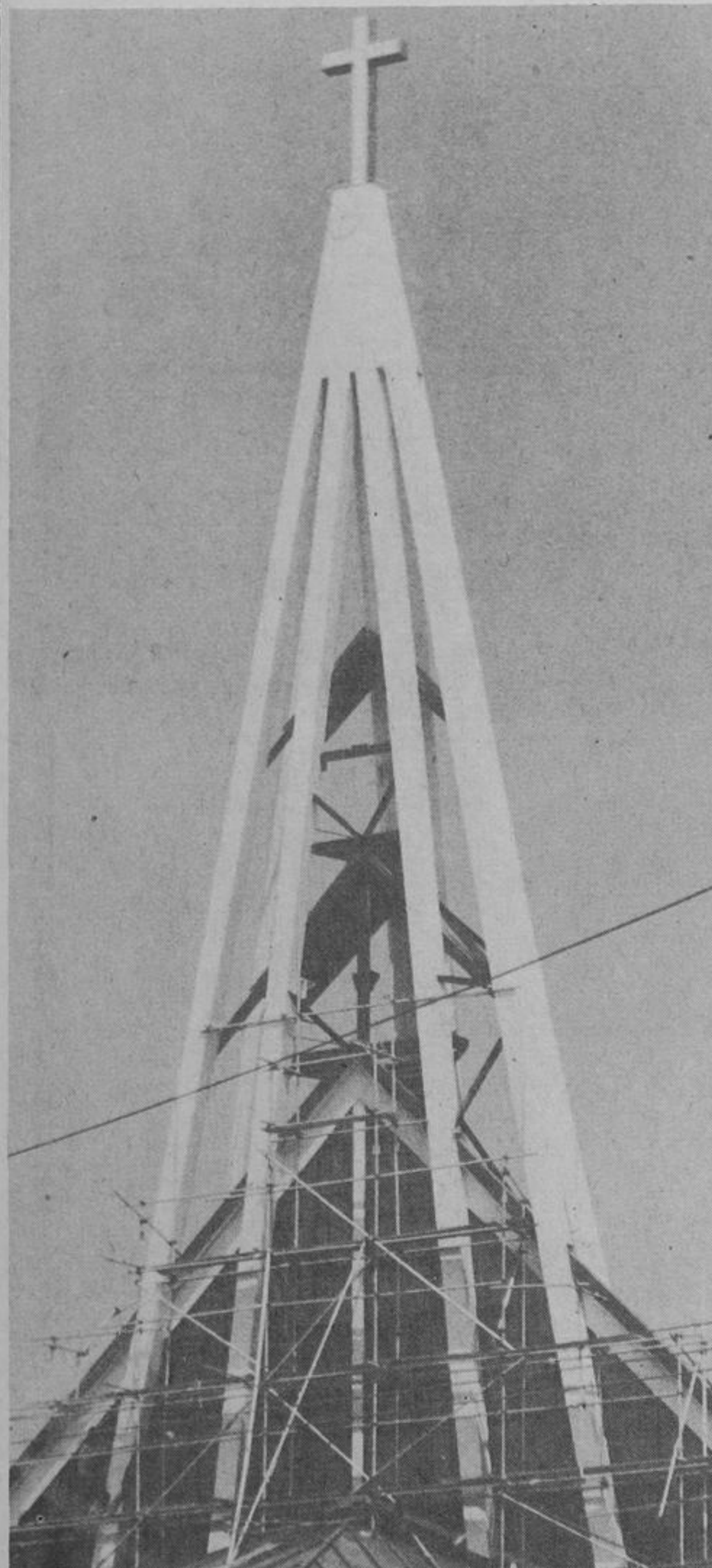
Repairs and renovations to the steeple atop St. Mary Immaculate Church in downtown Richmond Hill are continuing. Workers have a bird's eye view of the community from their lofty perch, several stories above the ground. (Liberal photo by Bruce Hogg)
