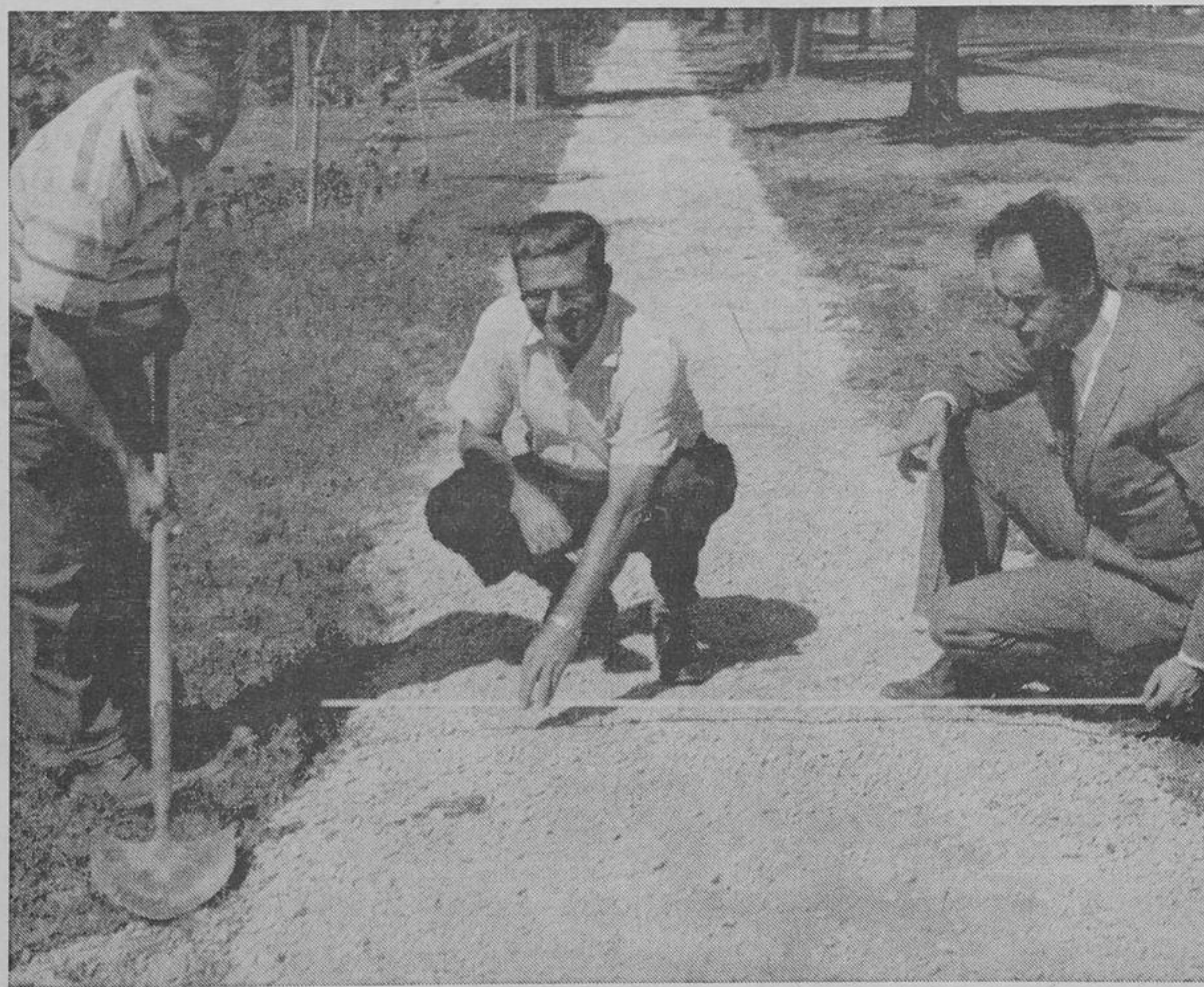
Inspecting the newly installed sidewalk on Bayview Avenue are left to right, Works Foreman Bob Bridges, Roads Superintendent Fred Bovaird and Assistant Works Commissioner Jack Vandermaas. Completion of the project is expected by the end of the week. (Staff Photo)
